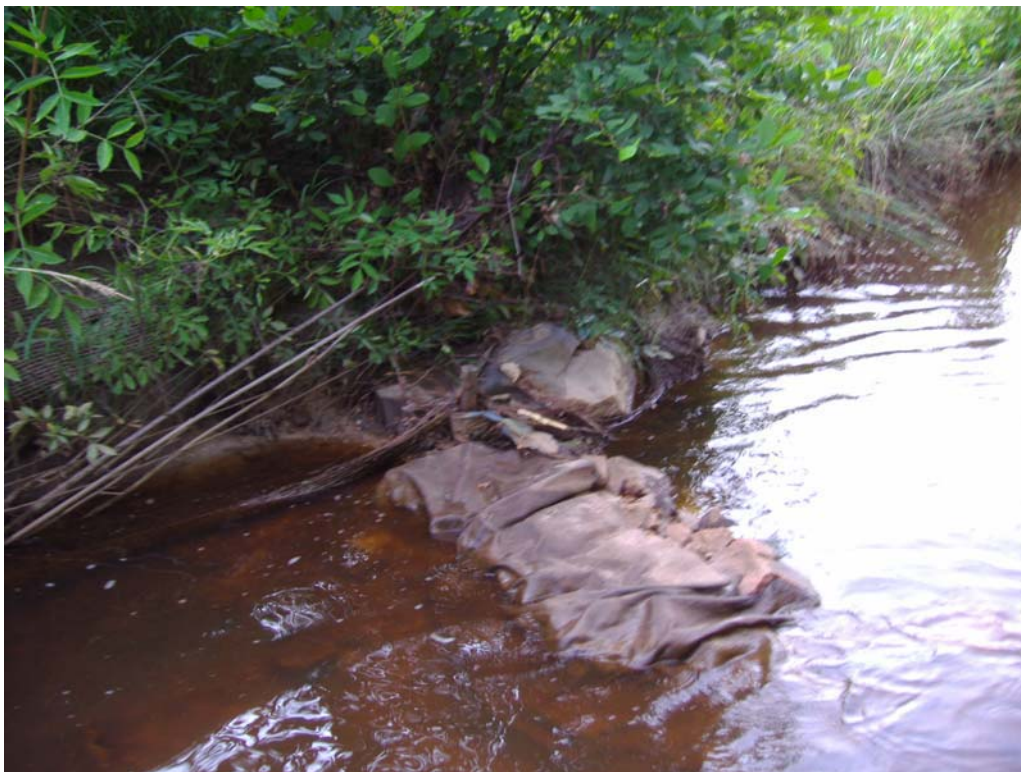
Photo 6. (SP 2-4, 16) Example of poorly built structure leading to structural failure and causing erosion on the banks (7/4/07)
