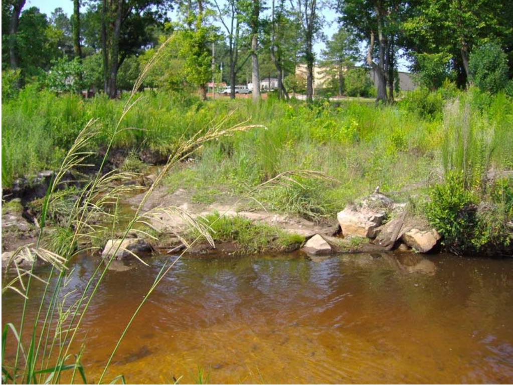
Photo 3. (SP 9) Outlet failure of the stormwater channel into the main reach (7/4/07)
