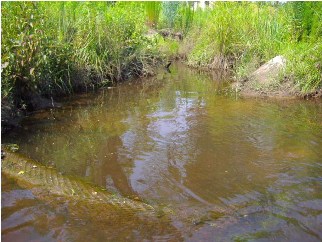
Photo 4. (SP 10) Outlet failure of the wetland pond into the main reach (7/4/07)
