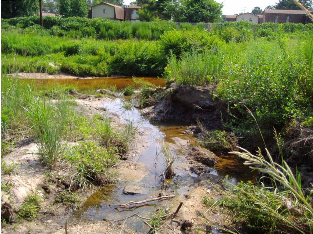
Photo 2. (SP 9) Bank erosion and migration of the design trapezoidal plunge basin (7/4/07)
