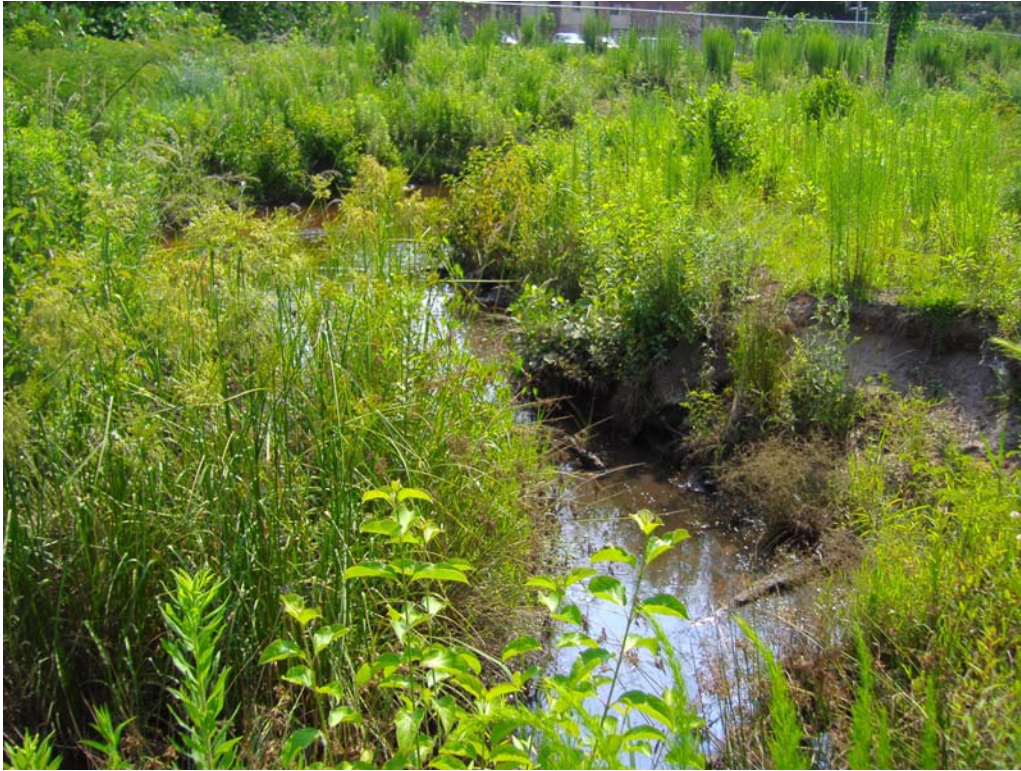
Photo 5. (SP 10) Bank erosion, migration, and failure of the wetland pond (7/4/07)
