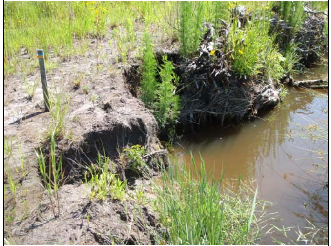
Problem Area 2, Station ~43+00
