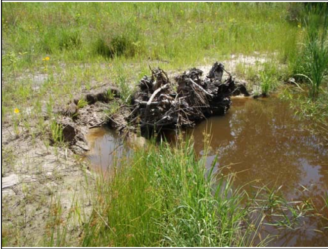
Problem Area 1, Station ~31+50
