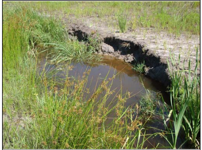
Problem Area 4, Station ~47+50
