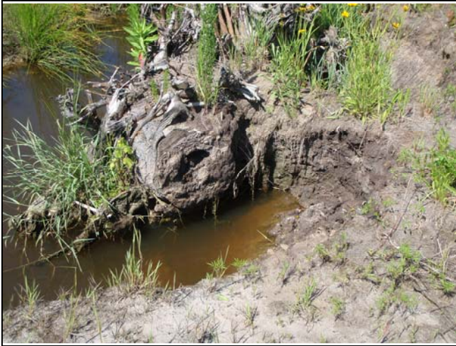
Problem Area 3, Station ~45+25
