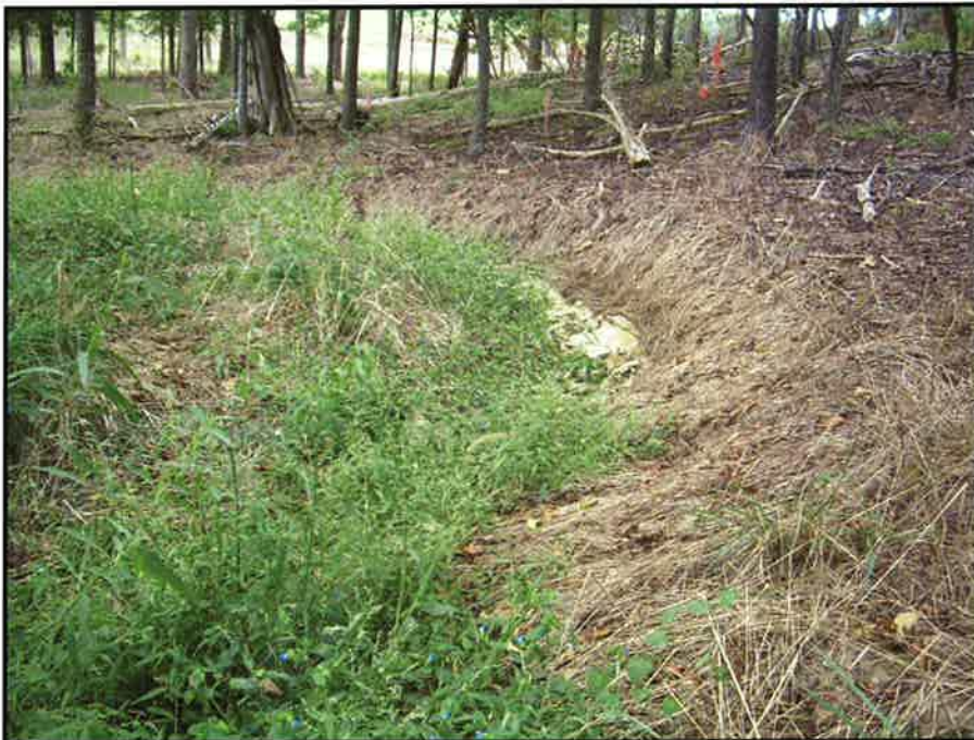
SPA 2 Bare banks along an outer meander bend on UT1 near station 5+50. Concern for stability if vegetation does not develop. (EMH&T, Inc. 9/19/09)
