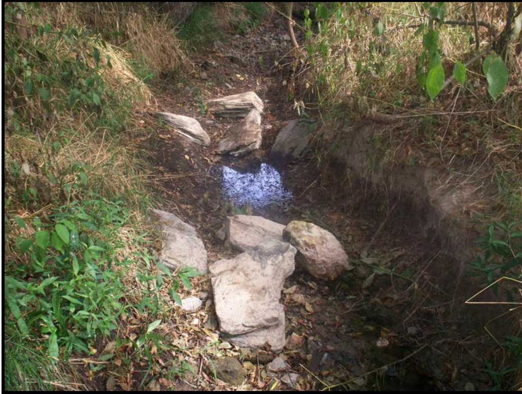
PA # 1 RCV structure failure. Boulders in mid-channel. STA 28+10 (South Trib.)
