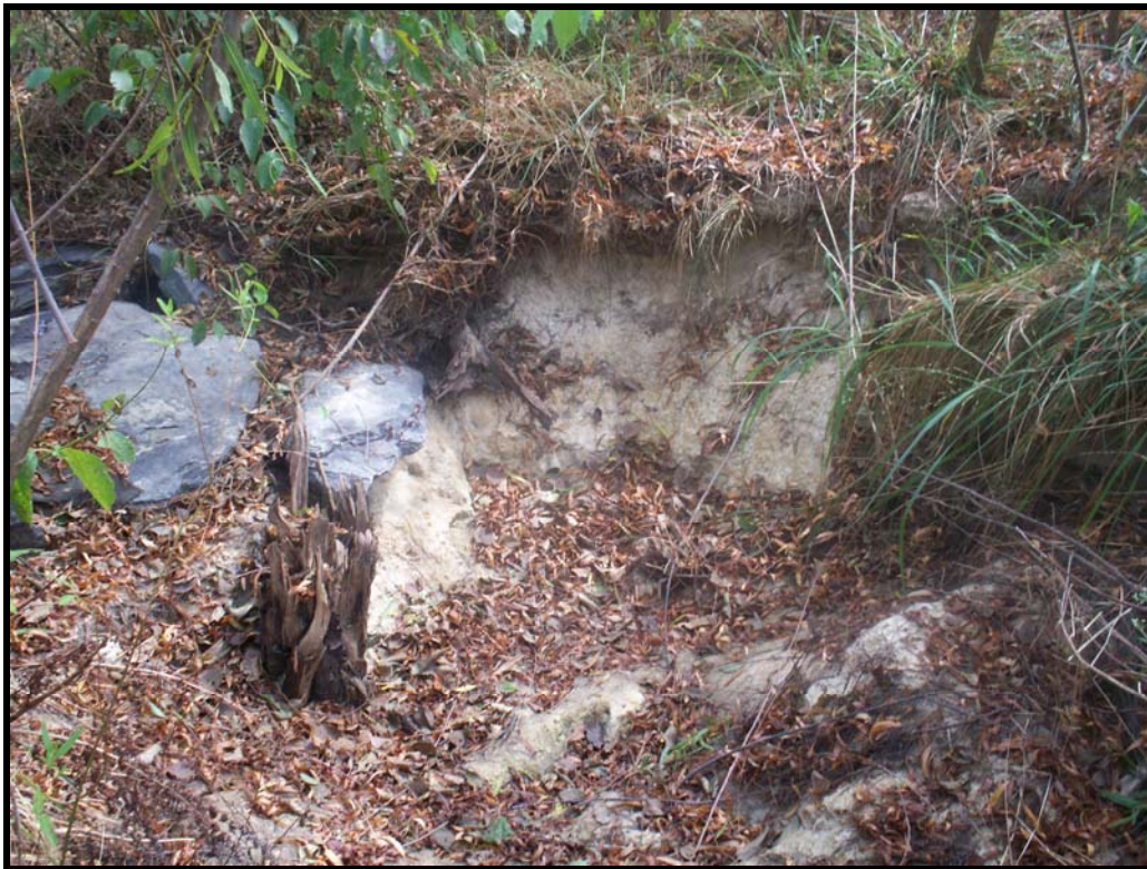
Pa #2 Right bank erosion @ STA 33+60 (South Trib.)
