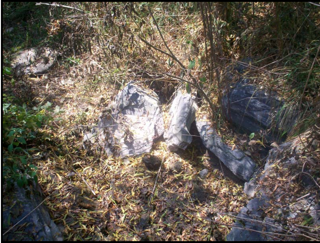
PA # 3 RCV structure failure. Boulders in mid-channel. STA 59+00 (North Trib.)
