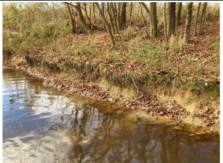
Meadow Branch, station 117+00 – Bank scour (11/02/2022)
