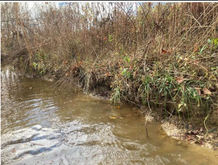
Meadow Branch, station 113+50 – Bank scour (11/02/2022)
