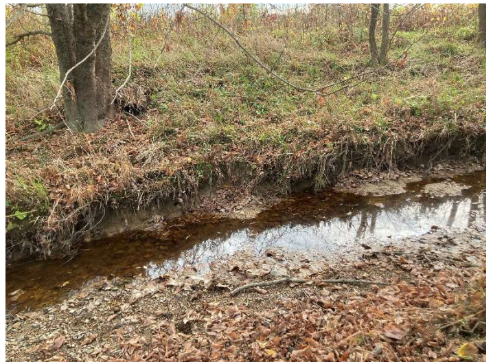
Meadow Branch, station 112+50 – Bank scour (11/02/2022)
