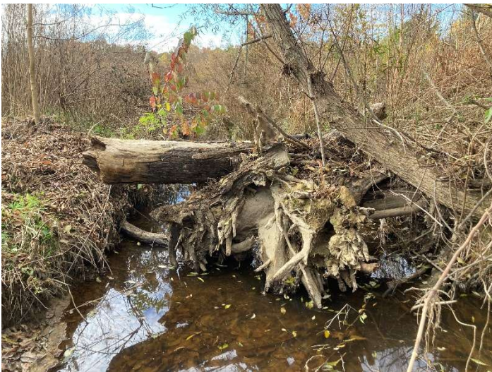
Meadow Branch, station 112+40 – Debris jam (11/02/2022)
