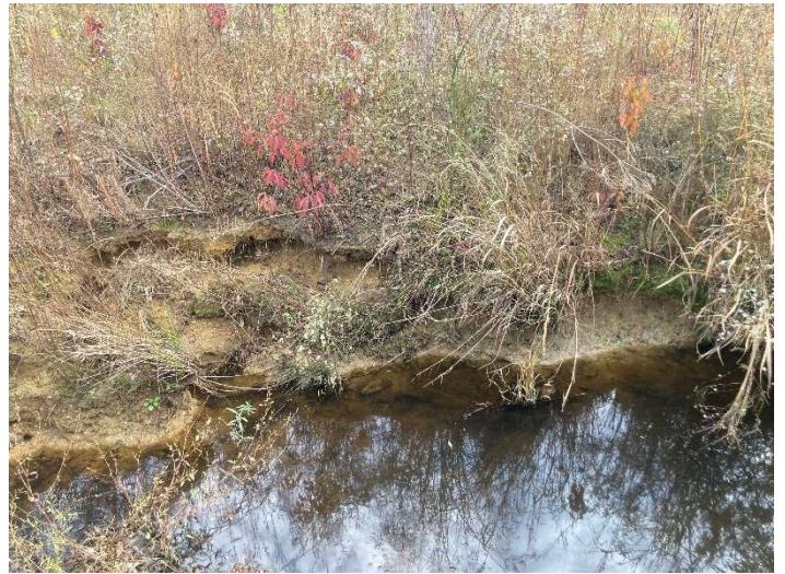
Meadow Branch, station 111+20 – Bank scour (11/02/2022)
