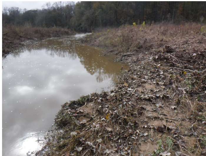
Issue: Structure washed out on Meadow Branch at station 103+50 (11/13/2020)
