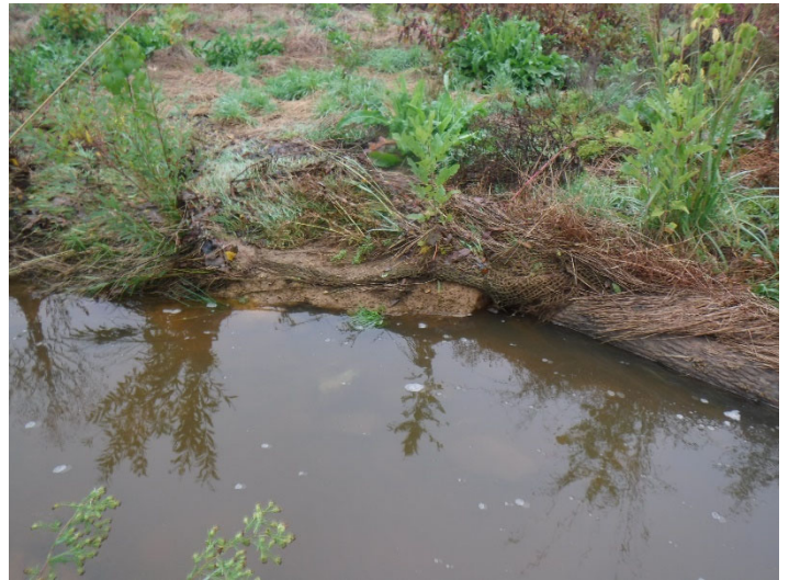
EF1 Slight Scour Right Bank Station 203+50 (11/13/2020)
