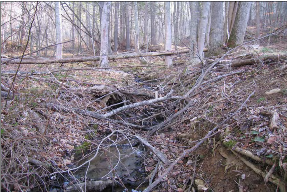
The beginning of T1-1 where a headcut has developed and the stream has become incised.
