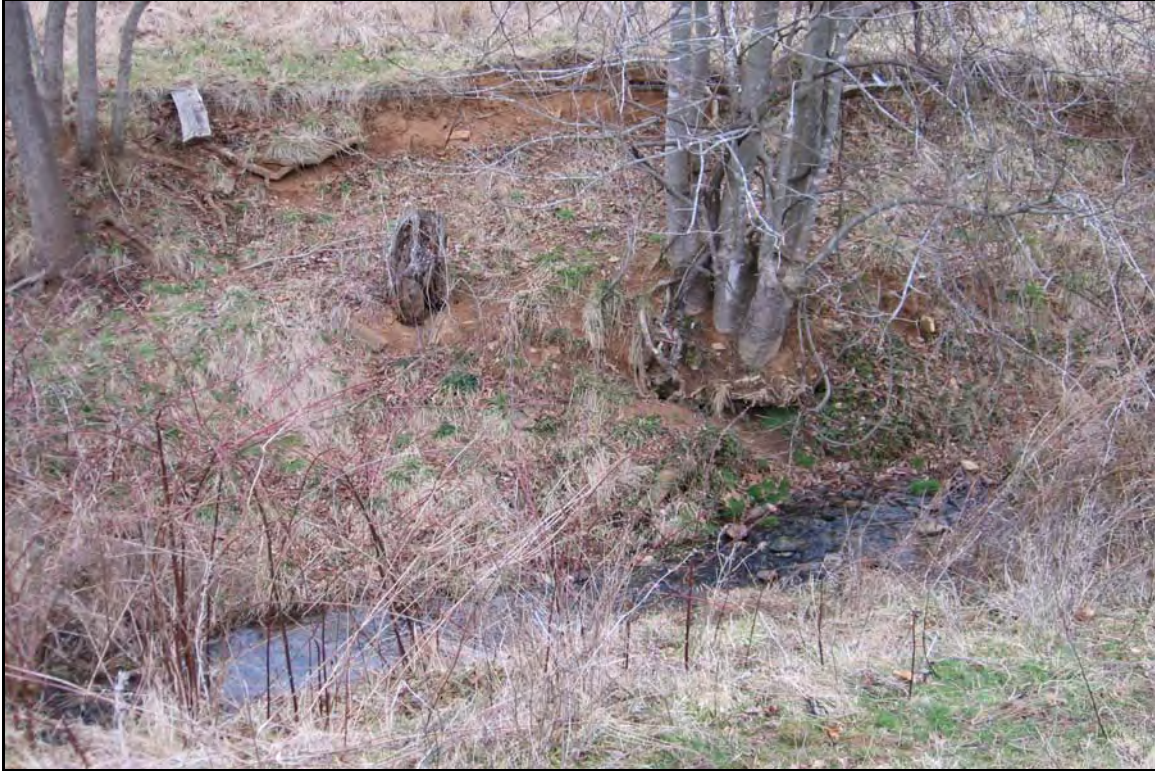
Looking down at WOC-4, which is entrenched within the valley in this section.
