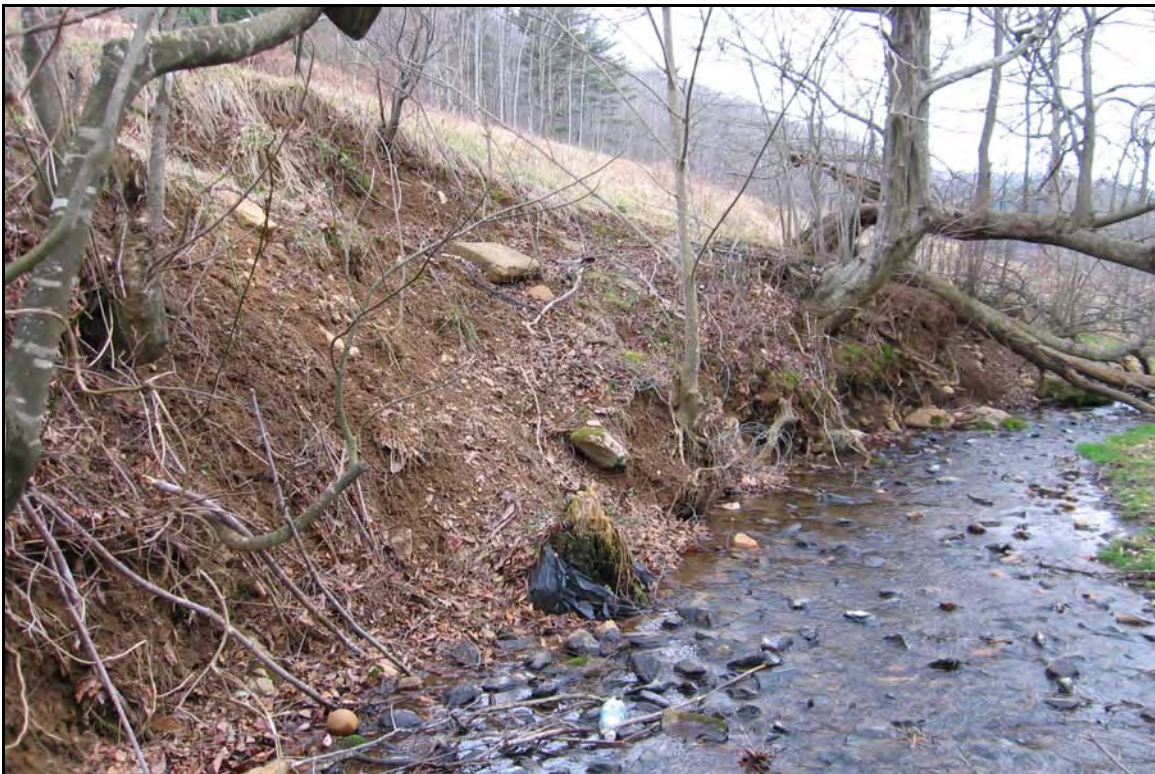
Bank erosion along WOC-4.
