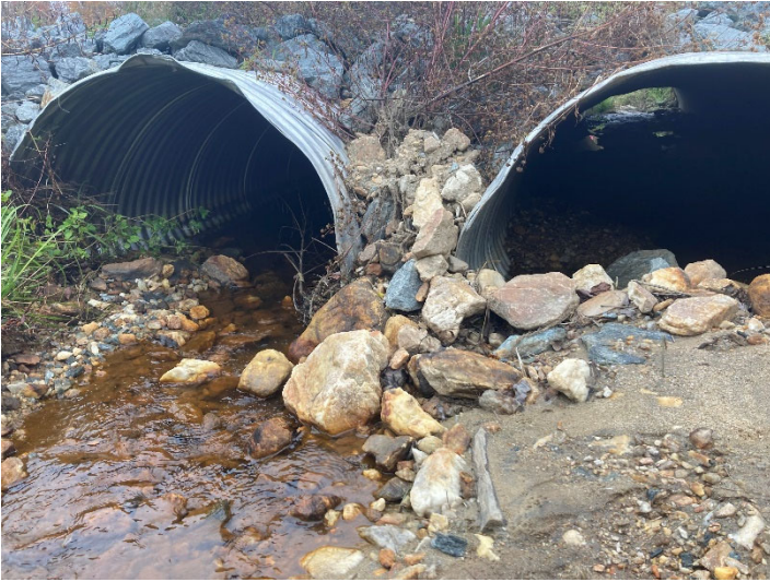
UT to Crab Creek R1 Crossing 2 (114+54) – Culvert Baseflow Adjustment for Aquatic Organism Passage (AOP) (10/12/2022)
