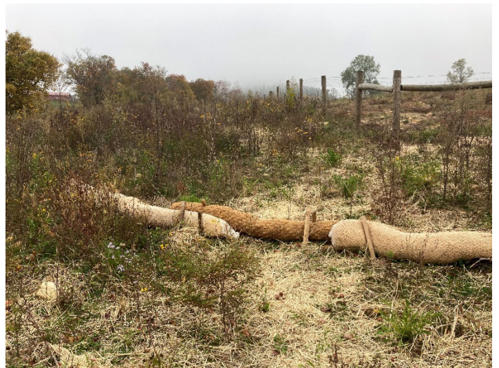
UT to Crab Creek R2/ UT4 Confluence– Coir Log Install to Mitigate Overland Sediment Influx from Area Outside of the Conservation Easement (10/12/2022)
