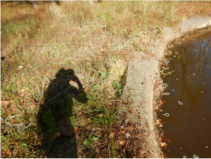
Before – Localized Erosion (11/4/2020)
