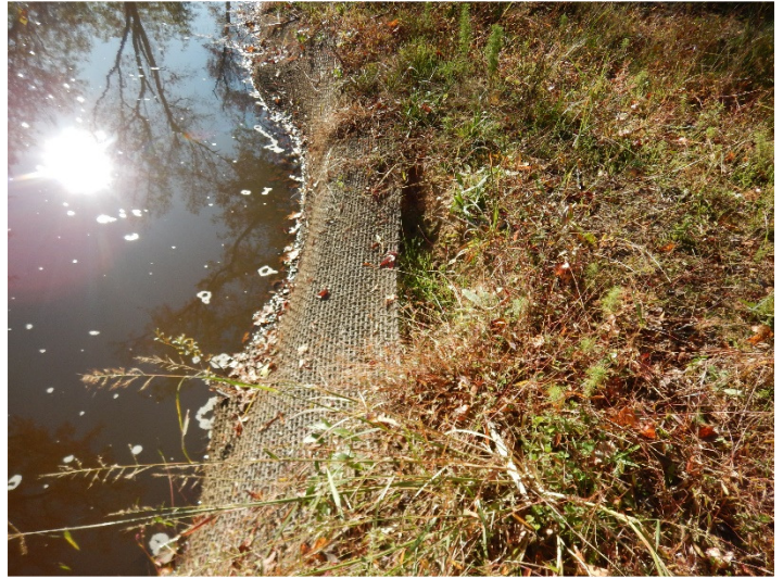
Before – Localized Erosion (11/4/2020)
