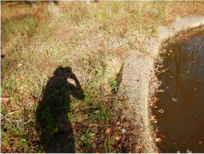
Before – Localized Erosion (11/4/2020)
