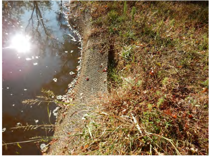
Before – Localized Erosion (11/4/2020)
