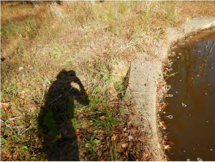
Before – Localized Erosion (11/4/2020)
