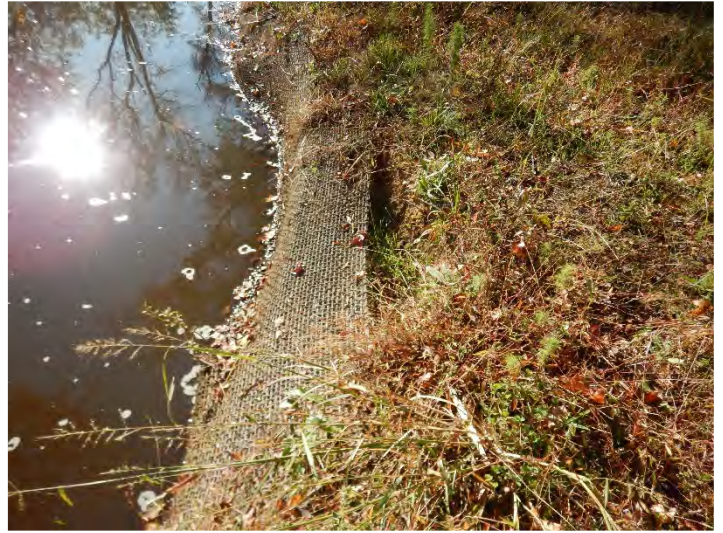
Before – Localized Erosion (11/4/2020)
