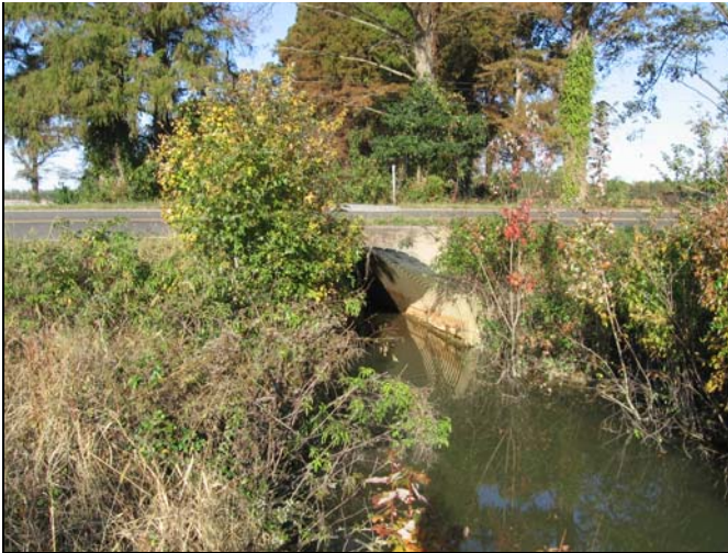
Culvert crossing under Kellogg Fork Rd (SR 1320) at beginning of project reach UT1.
