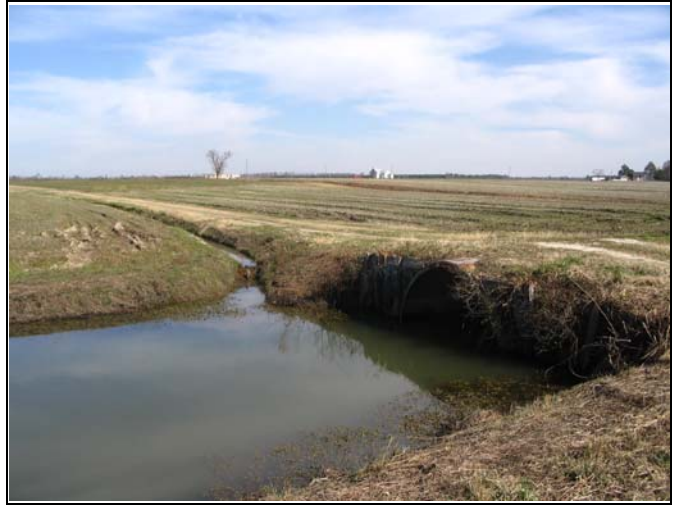
Farm access road at existing culvert crossing. Drainage ditch to be tied into proposed UT1.
