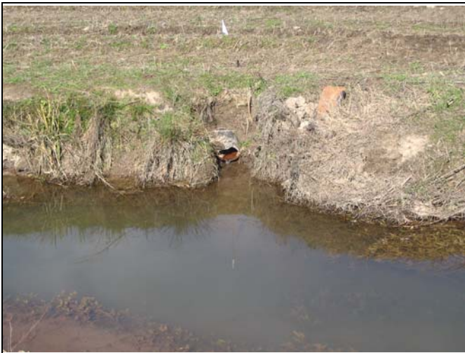
Example of existing drain tile to remain and tie into proposed stream and wetland areas.
