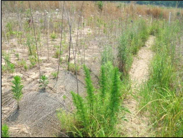
1. Poor Vegetation Cover-Main Channel Dula Thoroughfare (5/2008)
