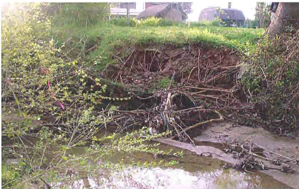
Eroded bank along last house before project ending boundary, Dye Branch lower reach.
