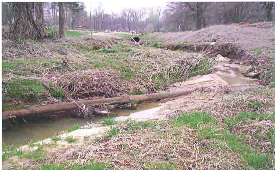
Old pipe in Dye Branch upper reach. Approximately 80 feet upstream of Mclelland Street culvert.
