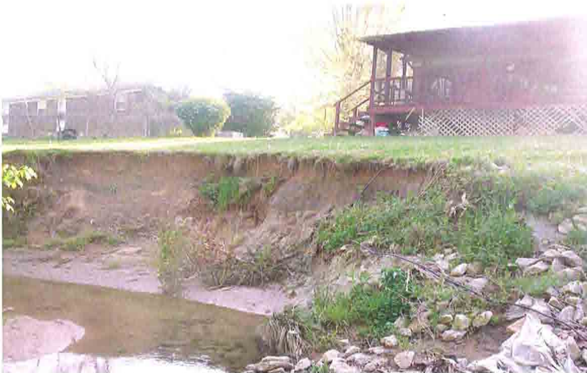
Eroded bank near Cabarrus Street, Dye Branch lower reach.
