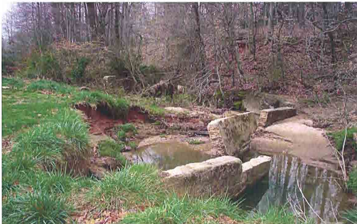
Concrete in stream on western side of basketball courts. Dye Branch middle reach looking downstream.
