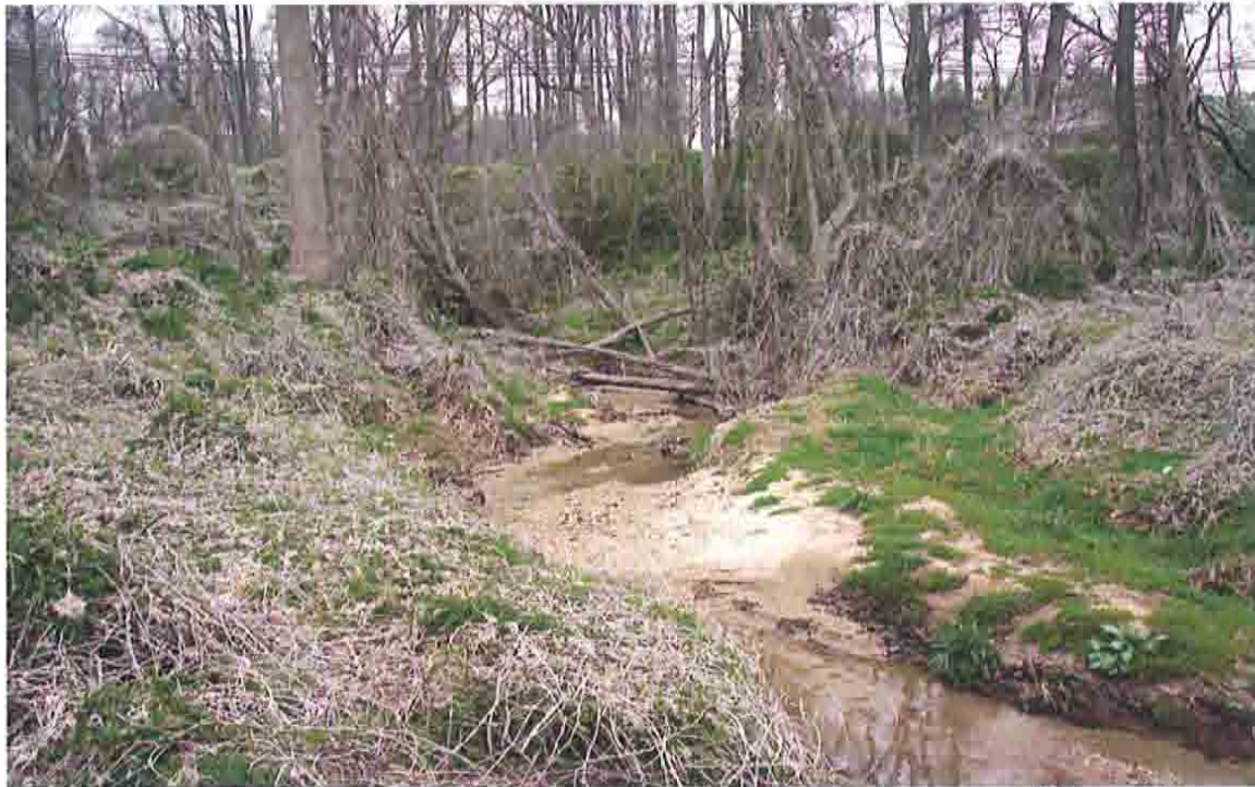
Debris in Dye Branch upper reach. Approximately 50 feet downstream of Center Ave.
