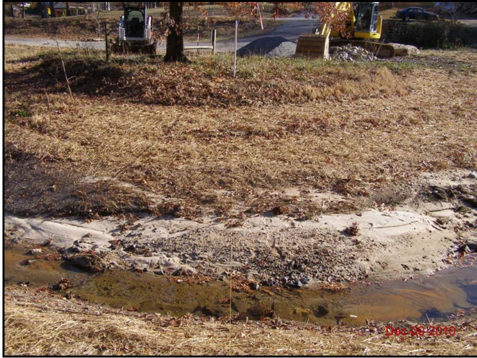
Dye Branch Upstream – Cross-Section 5 – Pool (Looking at Left Bank Descending) Baseline – December 9, 2010
