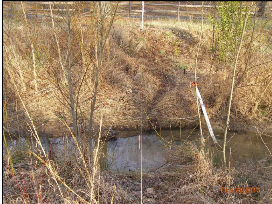
Dye Branch Upstream Reach – Cross-Section 4 – Riffle Right Bank Descending Monitoring Year 3 – February 28, 2013
