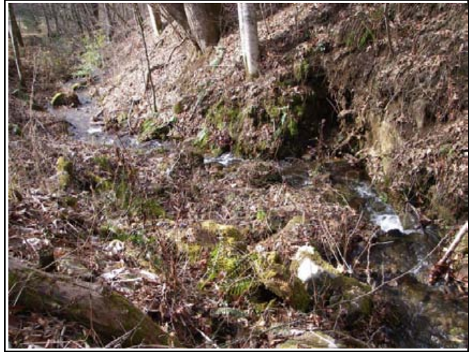
UT6 Reach 3 (enhancement) – Hillside erosion and bank slumping in sharp meander bend where channel is proposed for relocation away from valley wall.
