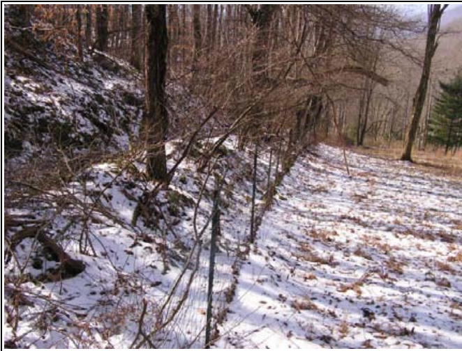
UT2 - Channel perched along the hillside with a berm along the right bank.
