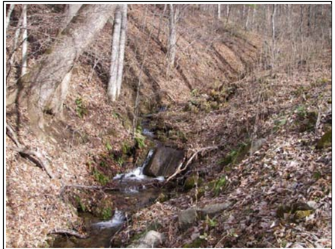
UT6 Reach 3 (enhancement) – Looking upstream at where channel will be relocated. Overwidened channel has eroded around existing grade control (boulder).
