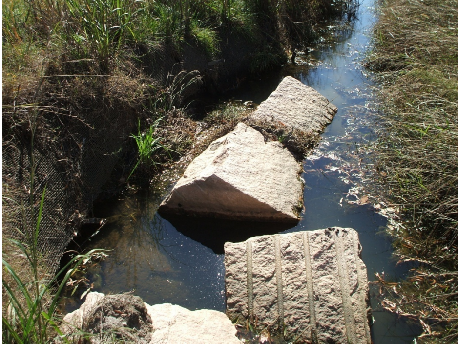
SP3 Reach 2 Station 21+ 50 Rock Vein Failure
