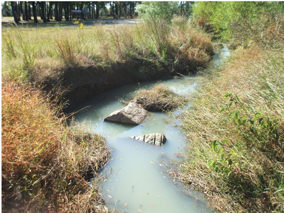
SP2 – Structure Failure - Sta. 21+50 - Reach 2
