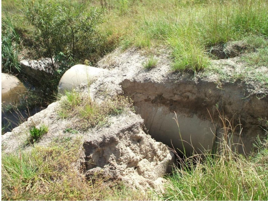
SP3 – Soil Erosion Station – Station 34+00 – Reach 2
