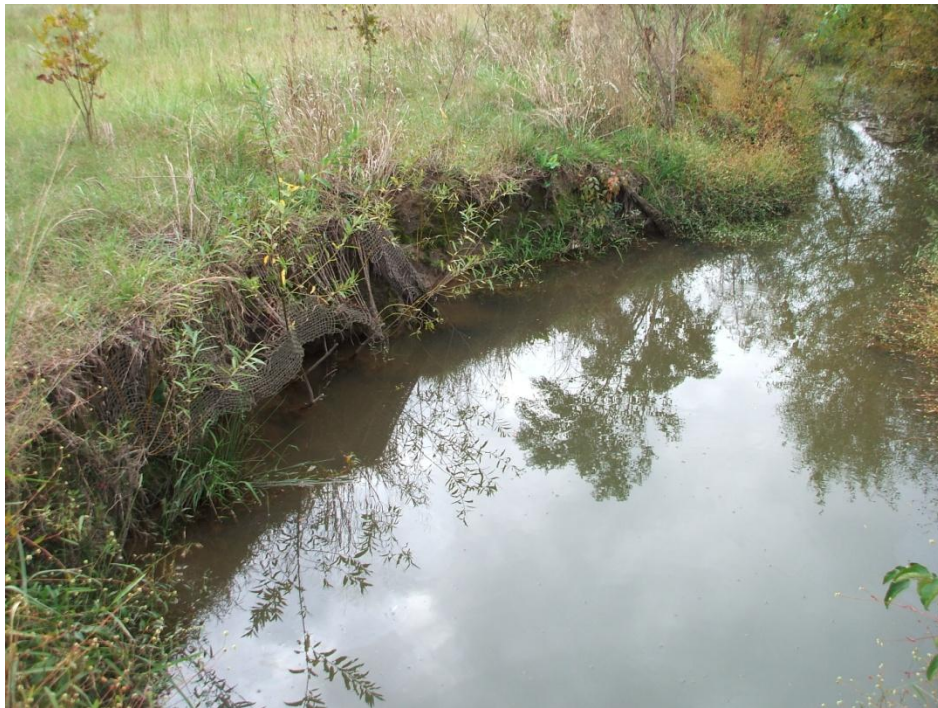
SP2 – Bank Erosion - Sta. 21+50 - Reach 2
