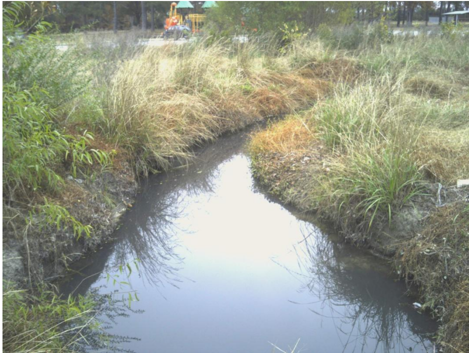
SP1 – Marginal bank erosion near culvert - Station 10+00 – Reach 2
