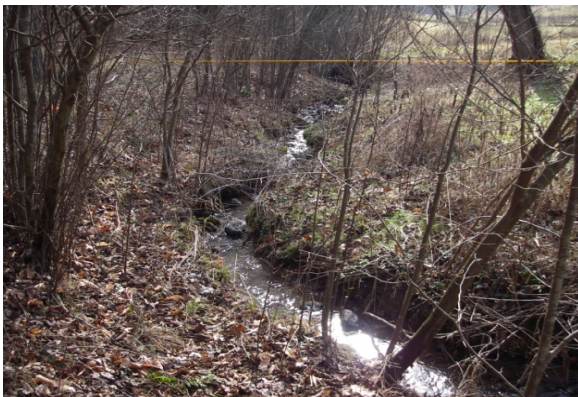
Elk Branch Reach 2, slightly incised and very narrow resulting in toe erosion
