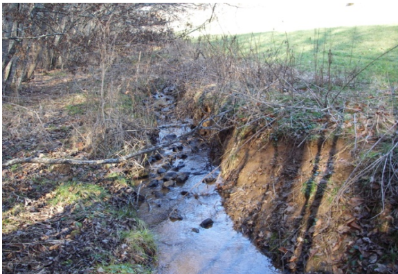
Bank erosion in Reach 1 of Elk Branch
