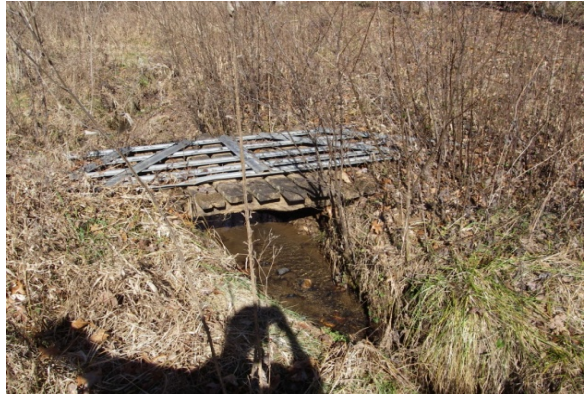
Footbridge between Reach 1 and Reach 2 of Elk Branch (location of easement break)
