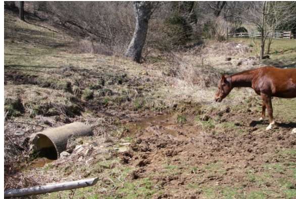
Location of proposed easement break, area to be repaired and culvert correctly installed for x-ing
