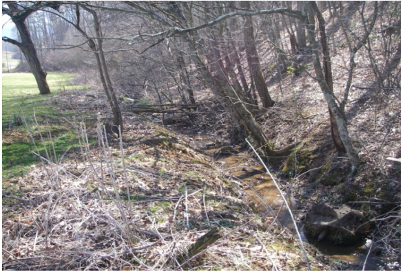
Channelized area against valley wall with leaning and fallen trees in Reach 1 of Elk Branch
