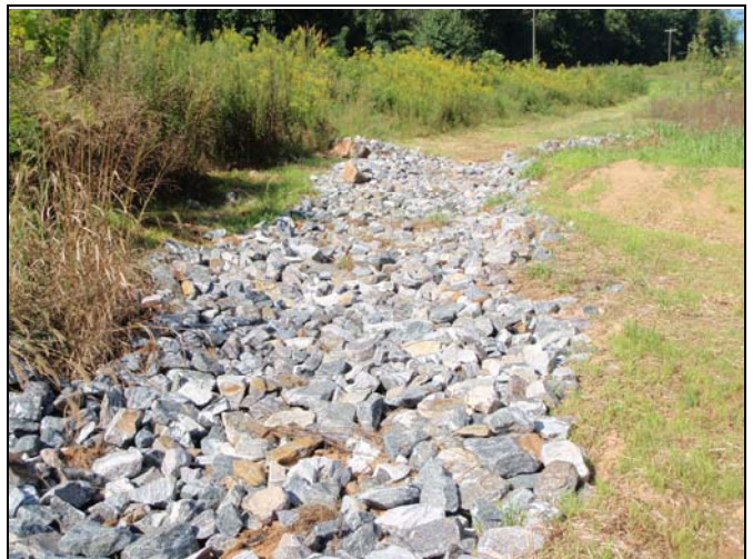
August 2009 - Repaired roadside swale using Class B stone, installed above and below the headcut
