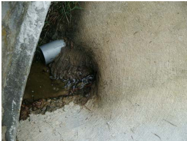
SP3 – Weir leak.
