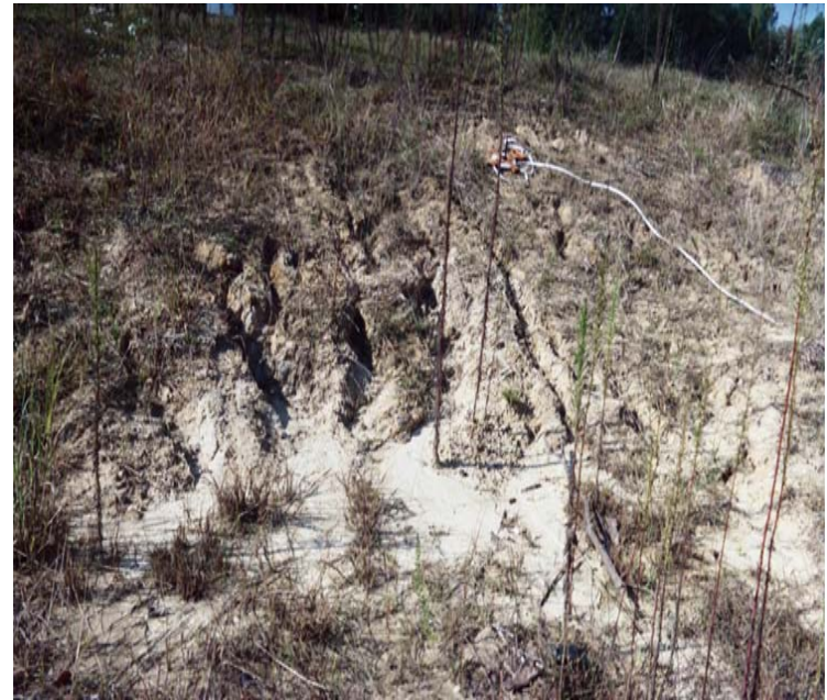
VP-2: Rill Erosion (STA34+00 to 34+25)
