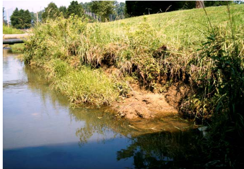
SP6. Bank undercut/scour
