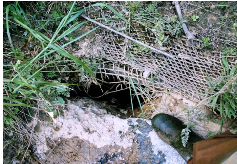
SP8. Vane backcut/scour
