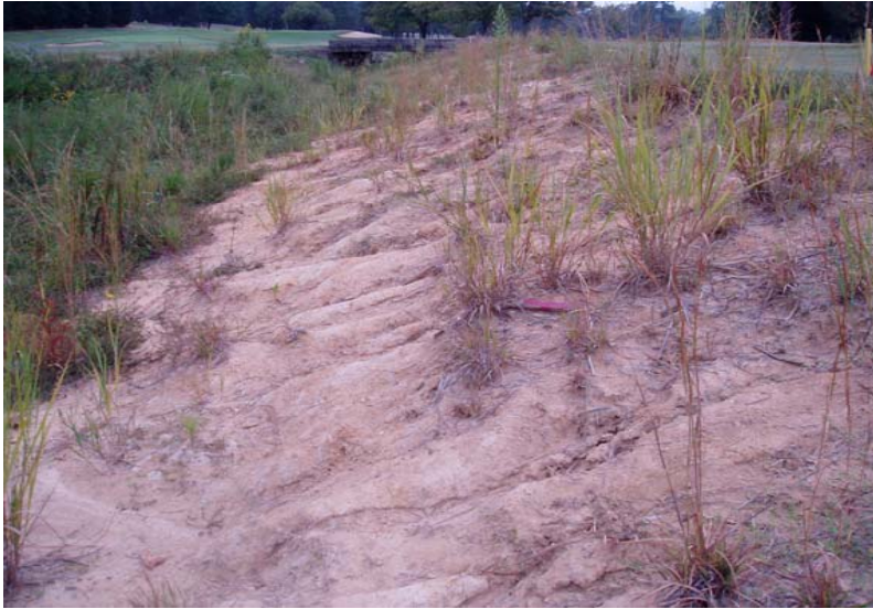
VP1. Bare soil/eroded slopes
