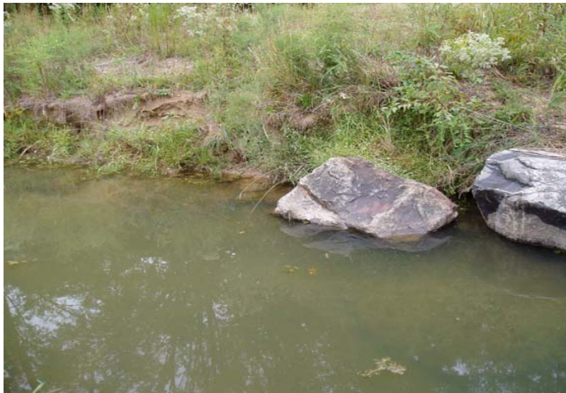
SP7. Boulder failure
