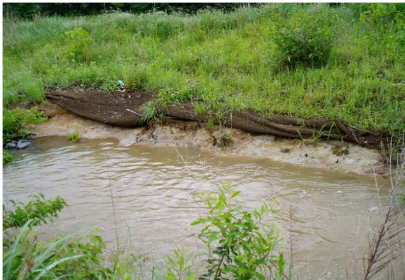
SP1. Scour with unattached matting (4/16/08)
