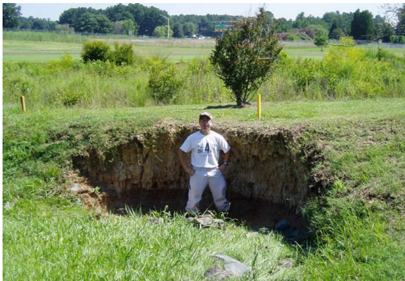
SP9. Scour in stormwater drainage (7/24/08)
