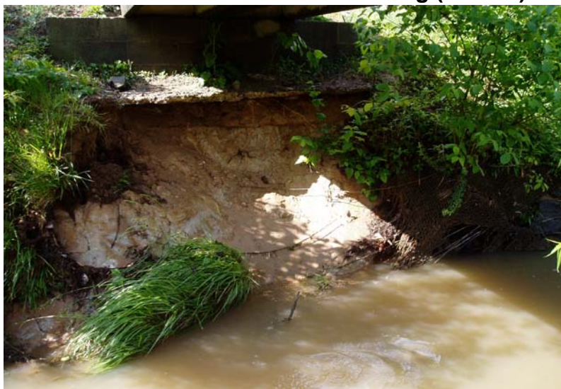
SP3. Bank scour under bridge (4/16/08)
