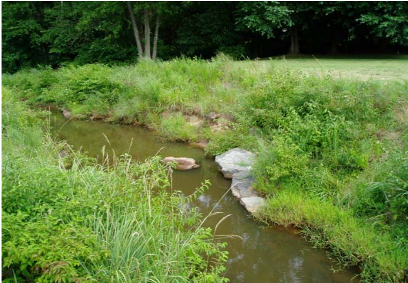
SP5. Scour at cross vane arm (7/16/09)
