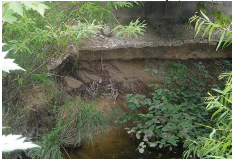
SP4. Scour under bridge footer (7/16/09)
