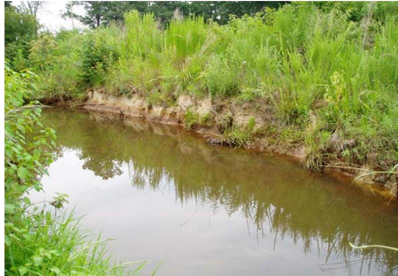
SP6. Bank slump/scour (7/16/09)
