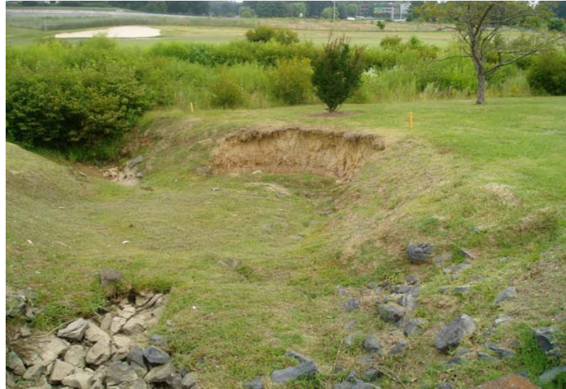
SP2. Scour in stormwater drainage (7/16/09)
