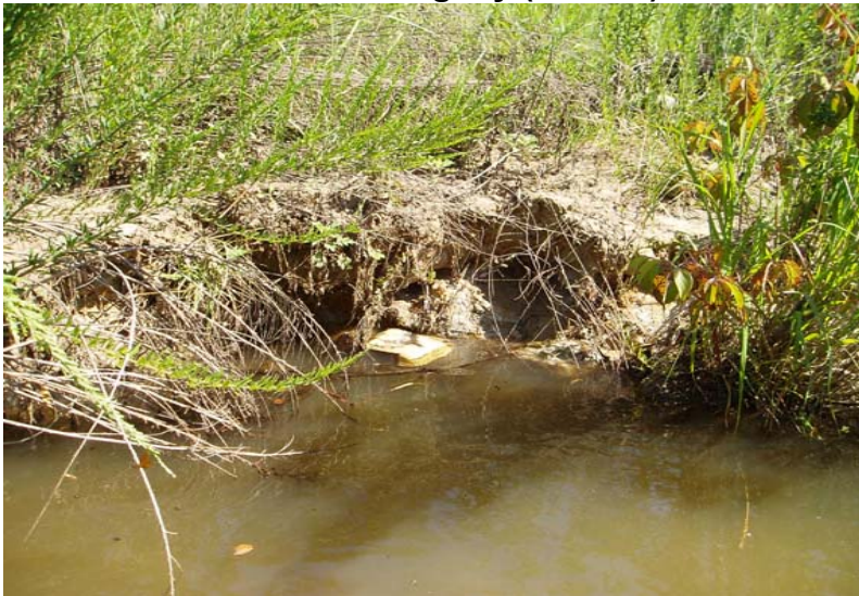
SP3. Bank scour (7/01/09)
