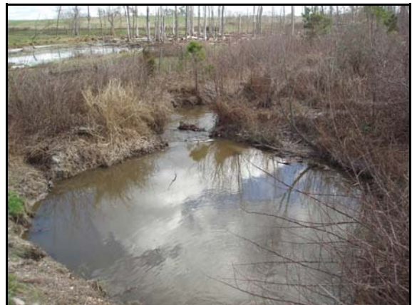
NPAC- Stream banks eroding downstream from culvert crossing
