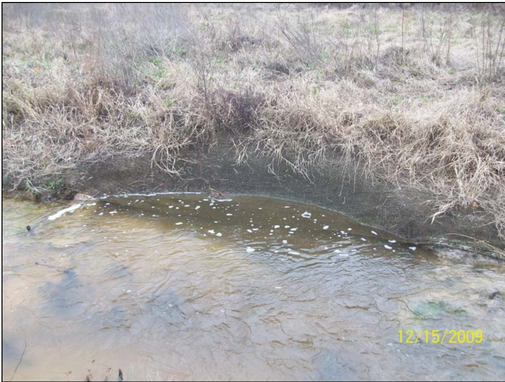
Bank erosion under coir matting near Station 56+60. MY01 – 12/15/09
