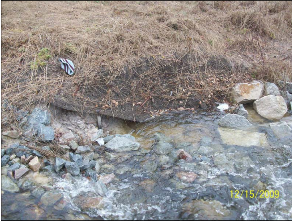
Bank erosion under coir matting near Station 12+50. MY01 – 12/15/09
