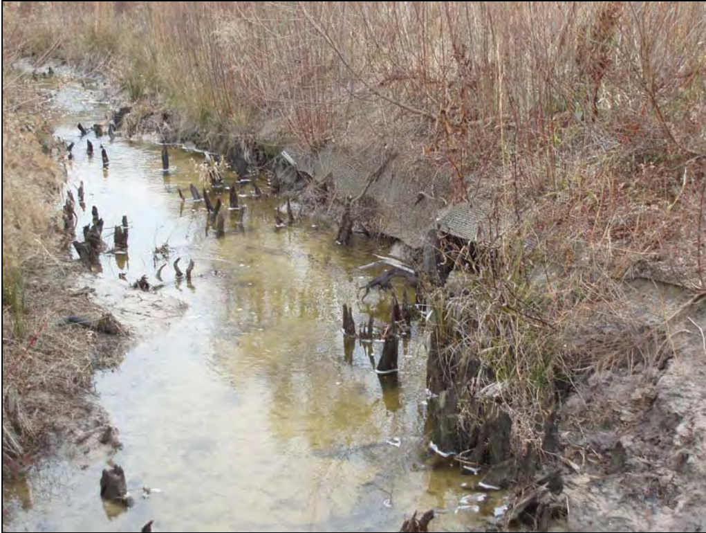
Erosion along toe of bank under coir matting near Station 60+75. MY02 – 12/22/10
