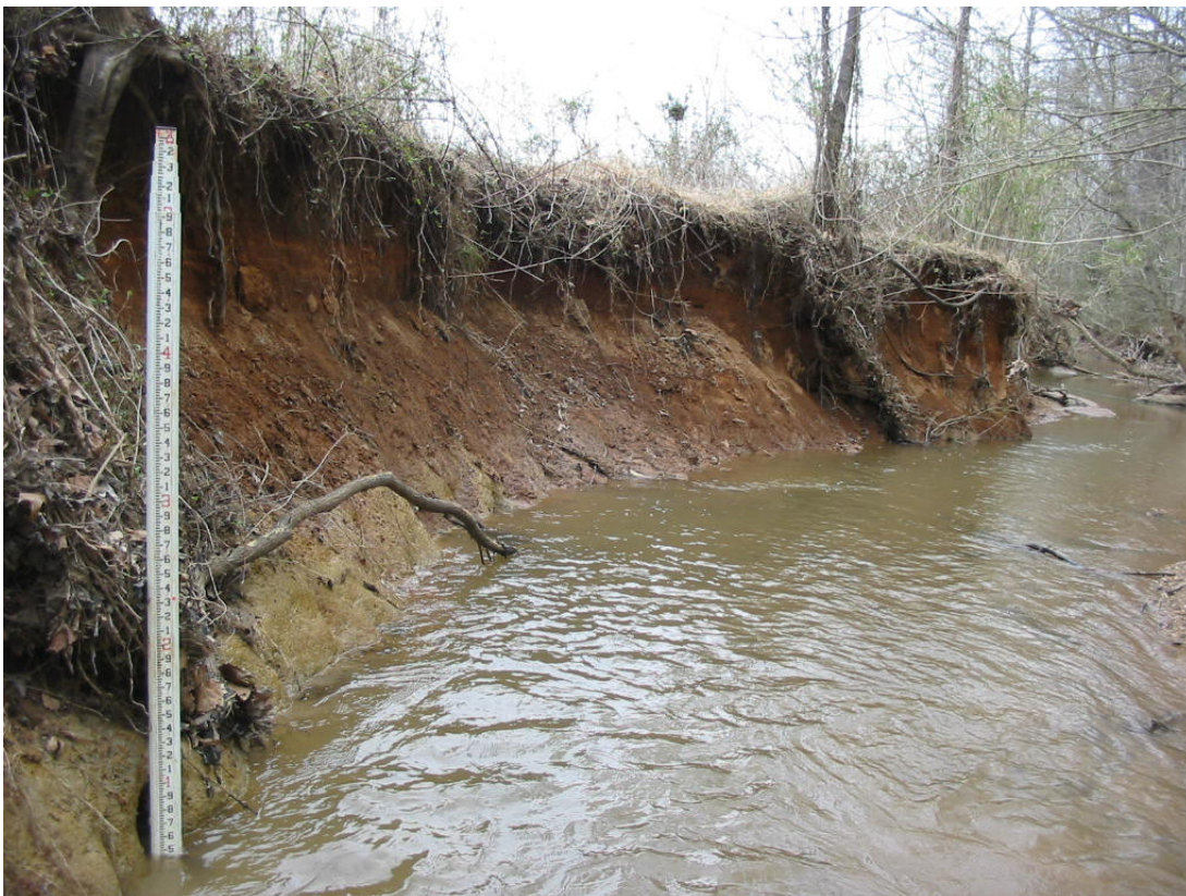
Photo 6: Eroding bank On Beaver Creek.
