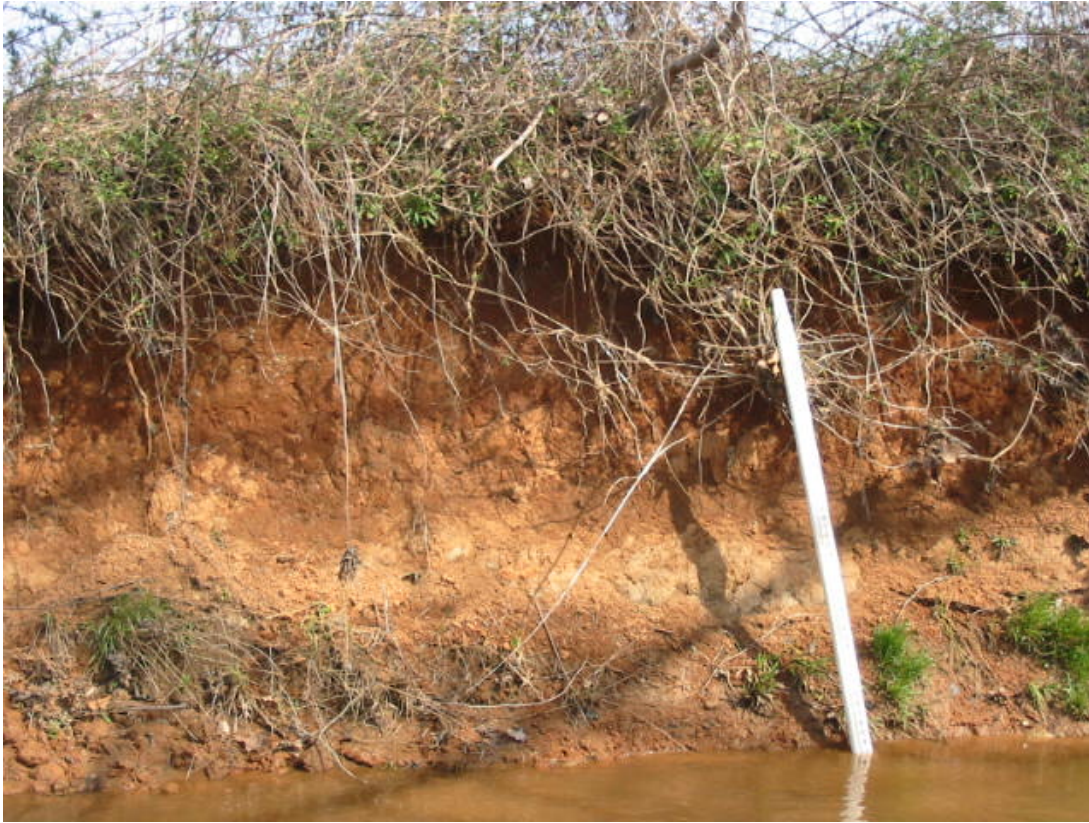
Photo 9: Eroding bank on Fifth Creek
