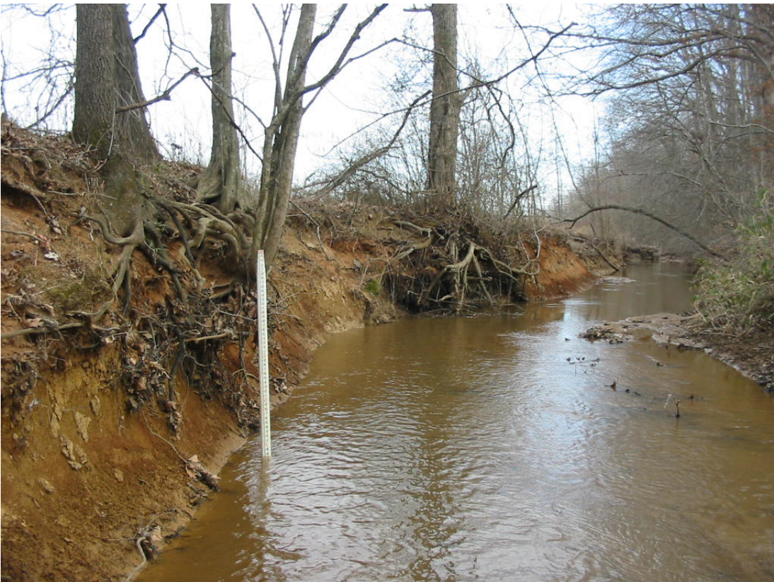
Photo 4: Eroding bank On Beaver Creek
