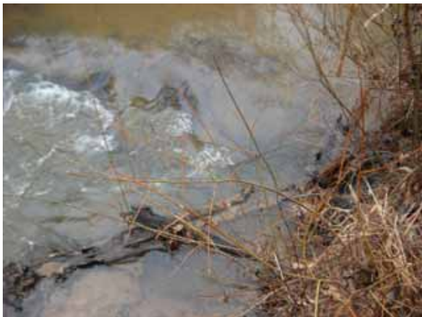
Photo Point 25. Cross Vane. Left arm scour. 12/5/13
