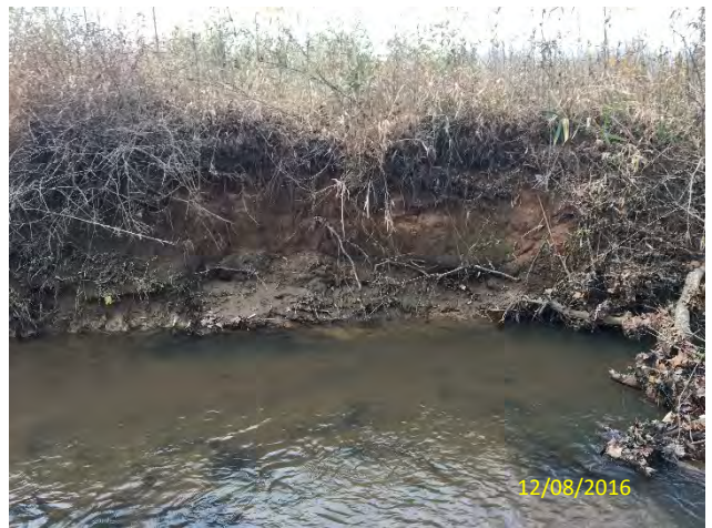
Bank Erosion 73+25 FTH
