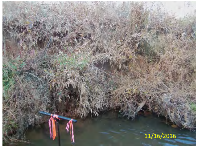
Bank Erosion 17+25 FTH
