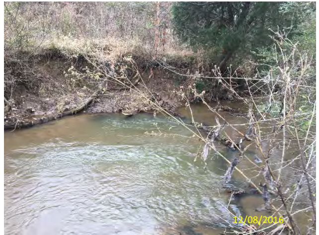
Bank Erosion 59+00 FTH
