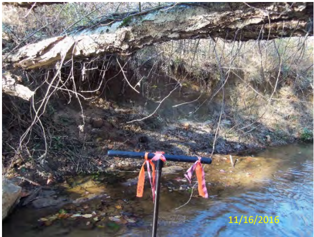
Bank Erosion 27+50 BVR
