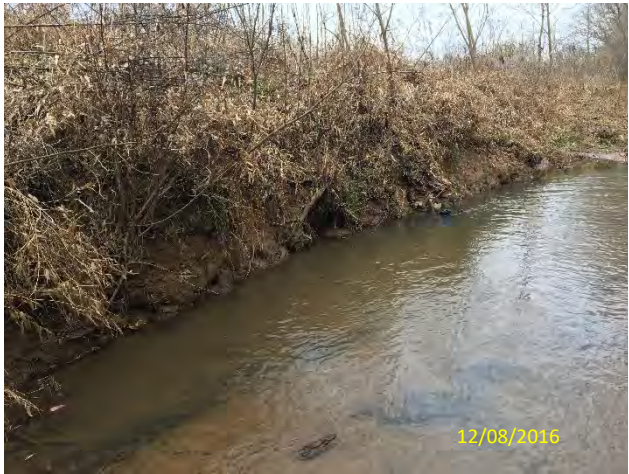
Bank Erosion 45+00 FTH
