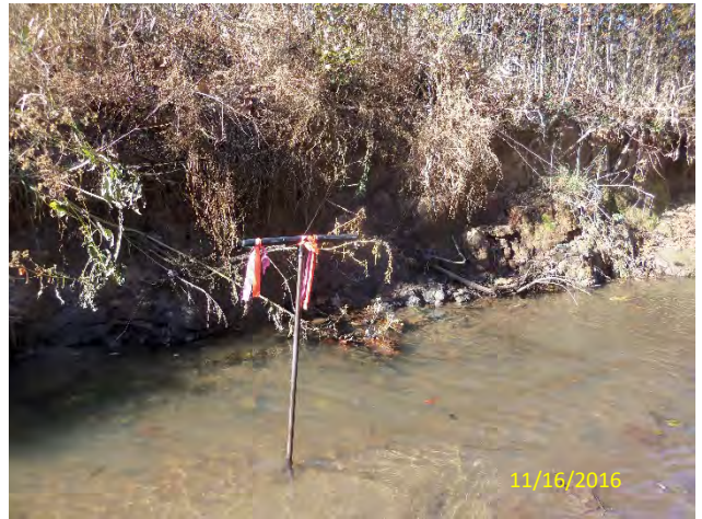
Bank Erosion 29+00 BVR
