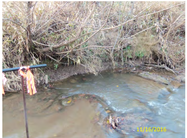
Bank Erosion 18+75 FTH
