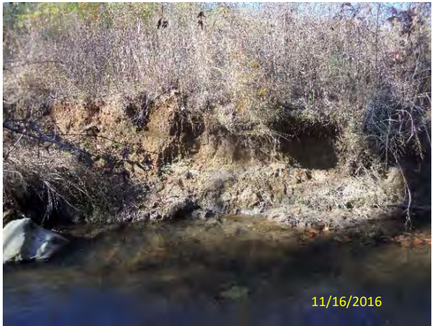
Bank Erosion 19+00 BVR
