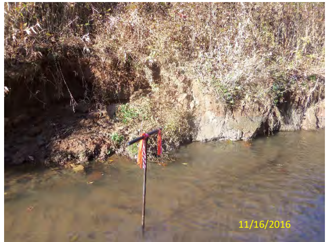
Bank Erosion 41+00 BVR
