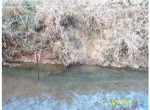
Bank Erosion 14+25 FTH
