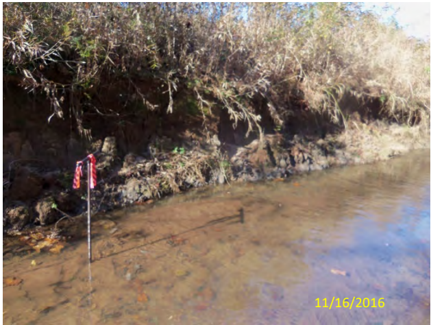
Bank Erosion 23+00 BVR
