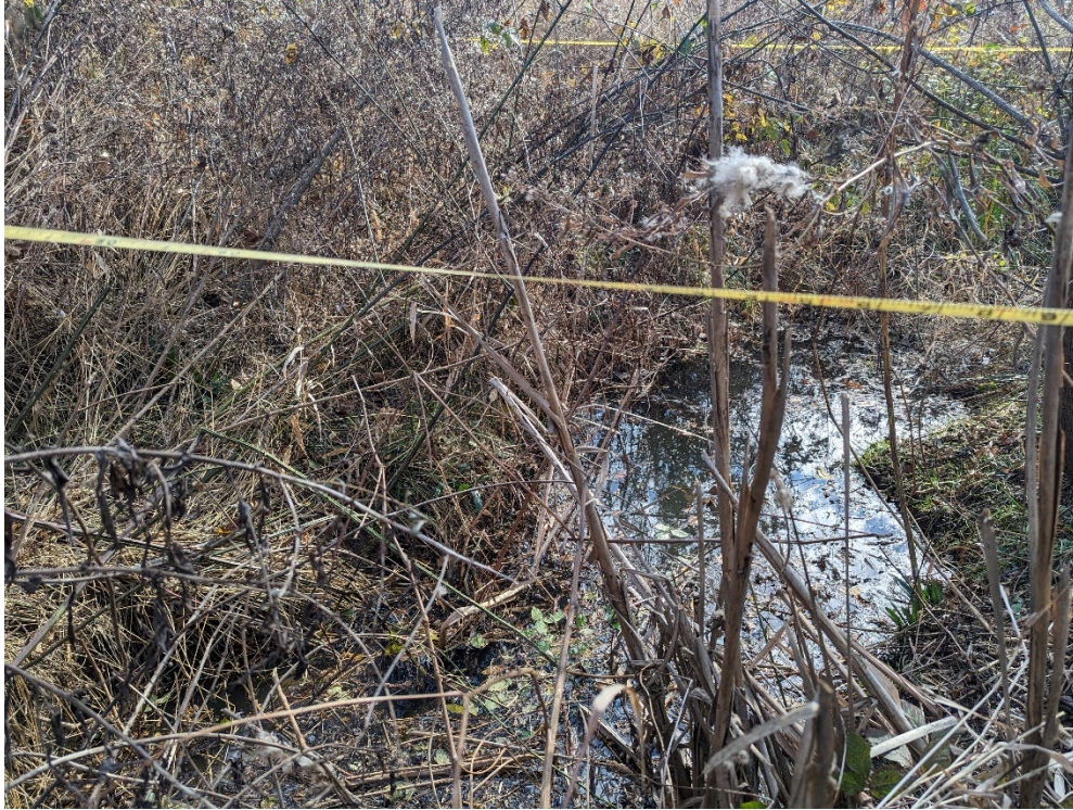
3. Cross Section 10, failed structure and extended pool, Station 133+50
