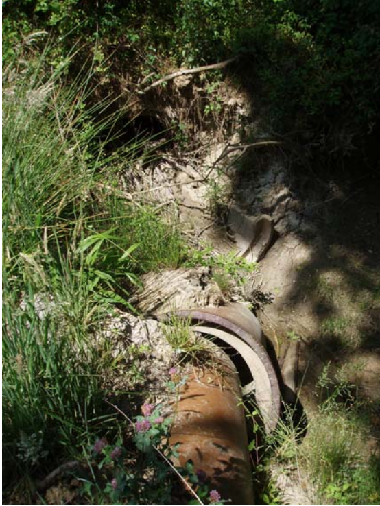
Photo 13 – Failed wastewater discharge outfall pipe in streambank, just downstream of the farm road crossing
