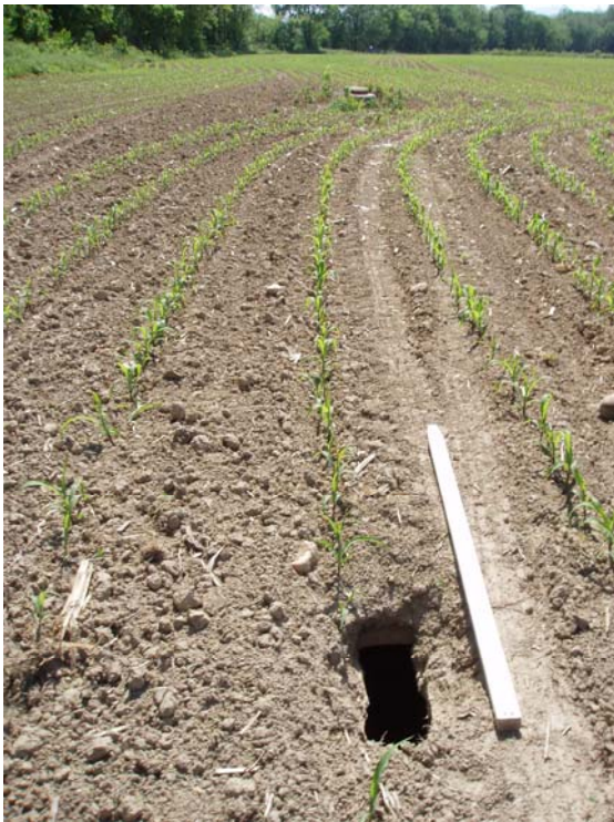
Photo 2 – Looking down the wastewater discharge outfall, with hole in the clay pipe in the foreground
