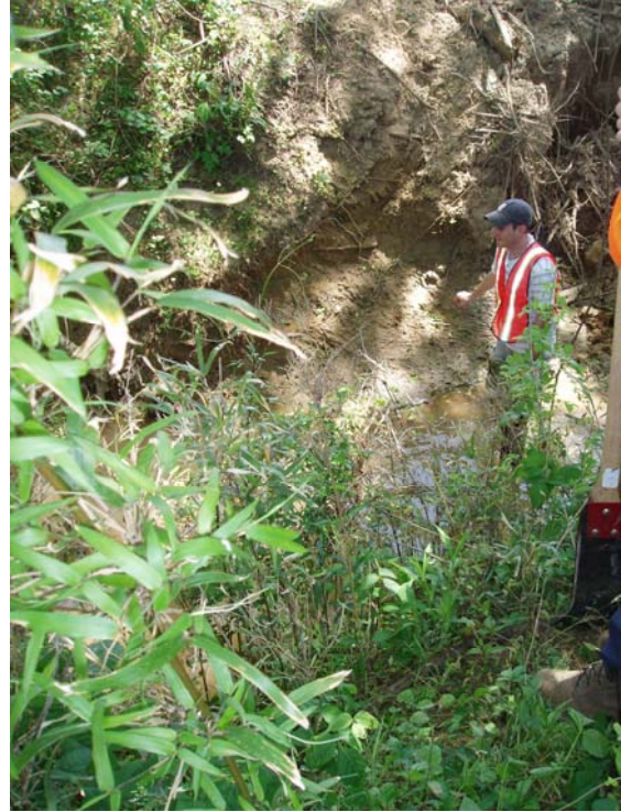
Photo 14 – Lower project reach, showing significant bank instability and channel incision
