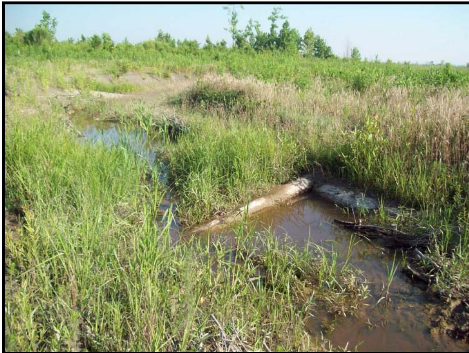
SPA6. Vegetation in channel behind bedded log structure; scour on right bank.
