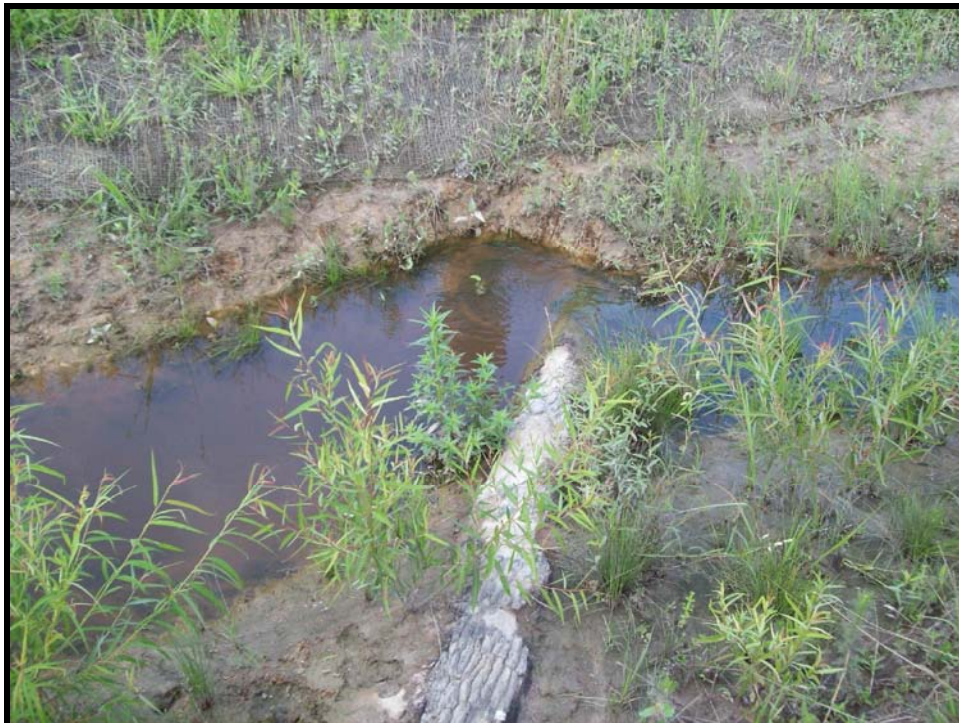
SPA2. Erosion behind bedded log structure due to improper installation.
