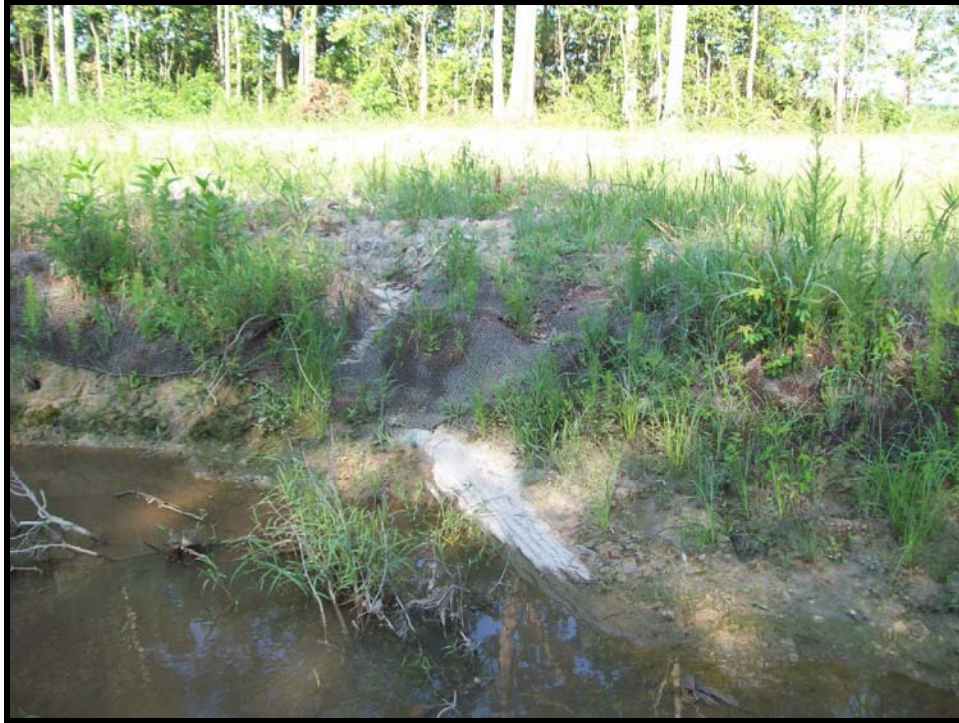
SPA7. Scour on right bank behind log vane.
