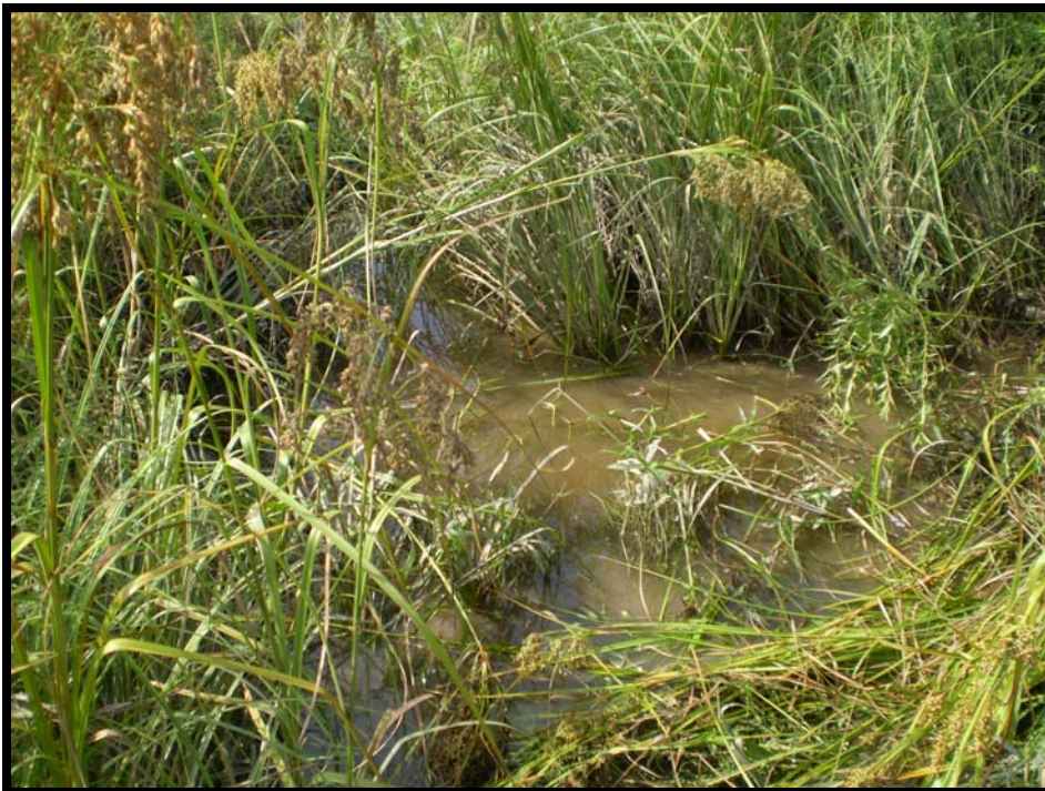
SPA4 – Scour around log weir @ station 46+50 (R3)
