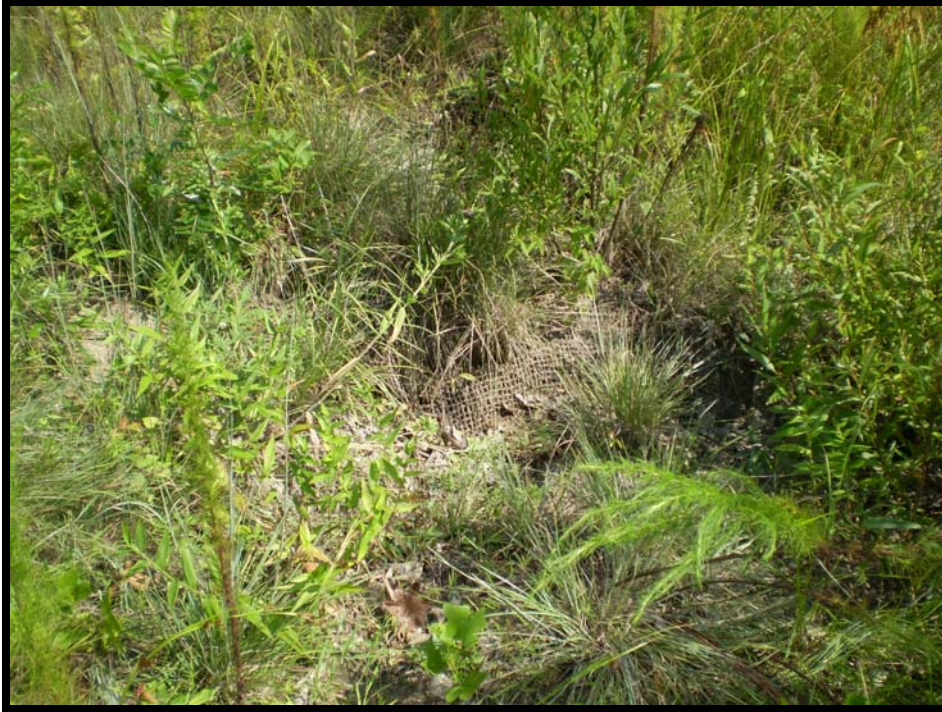
SPA7 – Scour behind log vane @ station 55+50 (R3)
