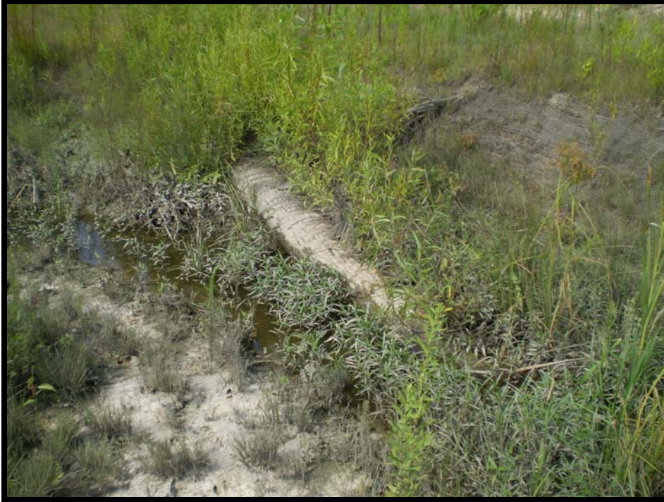
SPA5 – Heavy vegetation and scour behind bedded log structure @ station 49+30 (R3)
