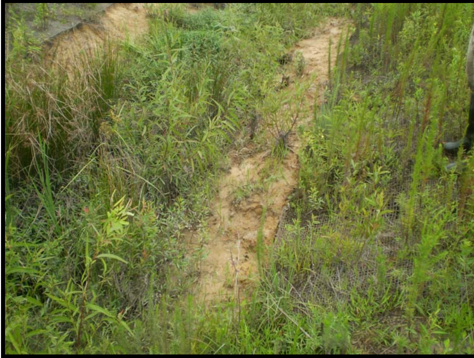
SPA1 – Minor scour on left bank @ station 9+75 (R1)
