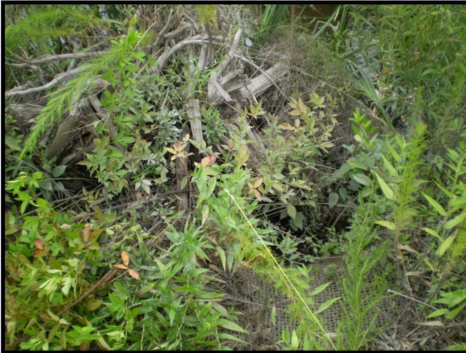
SPA2 – Erosion behind root wad @ station 12+75 (R1)
