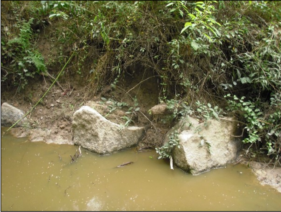
Stream Observation Area #5 – STA 78+80. Boulder toe is functional but bank above toe boulders is unstable and un-vegetated.
