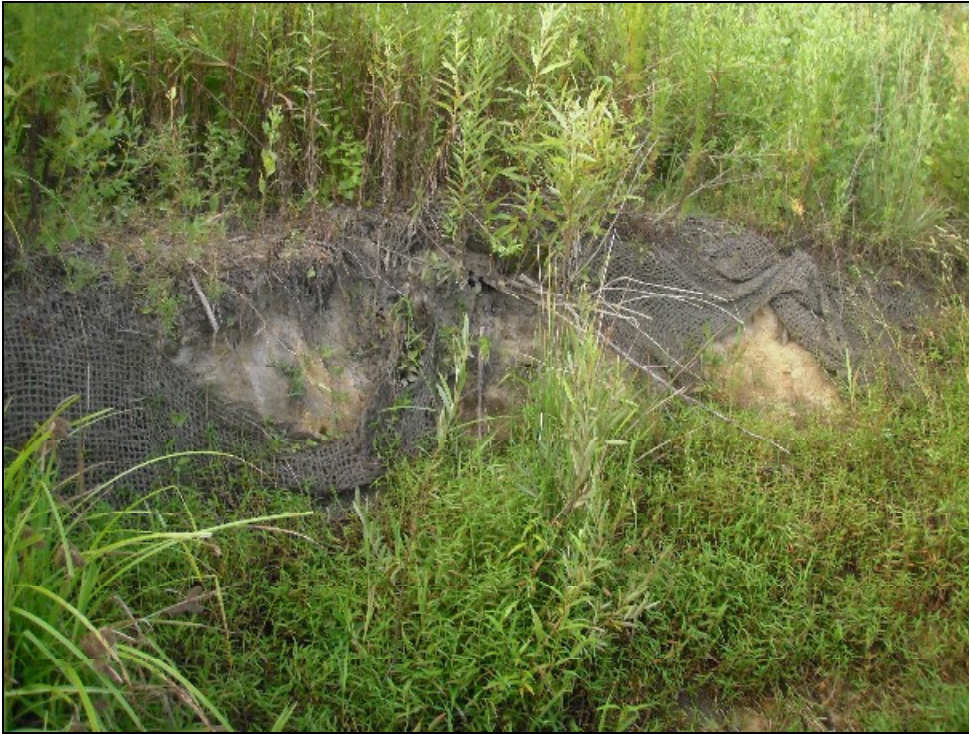
Stream Observation Area #1 – STA 9+80 – 11+50. Minor erosion and sparse vegetation behind and below matting due to clayey soils.
