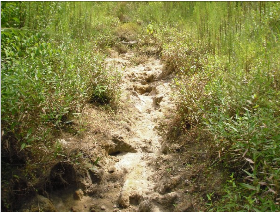
Stream Observation Area #2 – STA 73+70 – 74+40. Bed erosion likely due to improper slope at construction.
