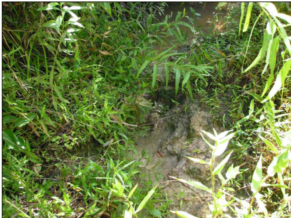
SOA #2 - Station 73+70, minor headcut with erosion
