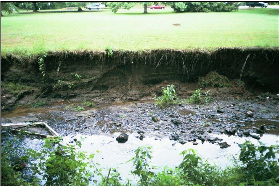
Severely eroded streambank. (Right bank at Sta. 11+50.)
