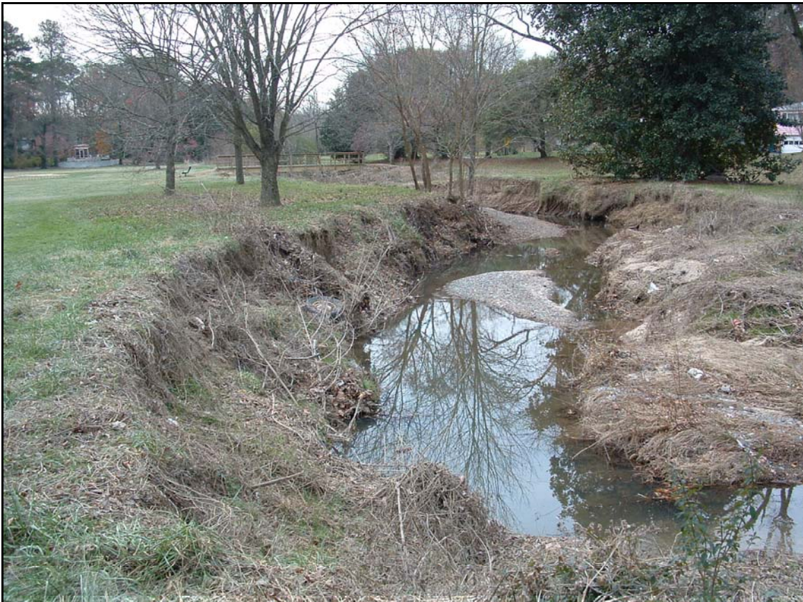
Typical degraded section in downstream project area. (Sta. 34+00, looking downstream.)
