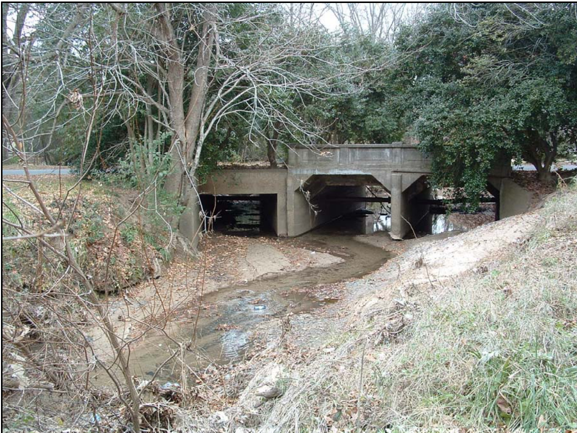
Second East Forest Hill Drive stream crossing box culverts. (Sta. 30+00, looking downstream.)
