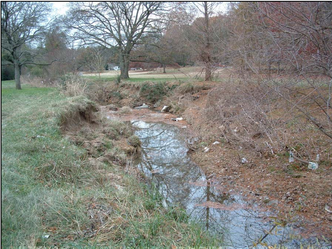
Typical degraded stream section in upstream project area. (Near Sta. 15+40, looking downstream.)
