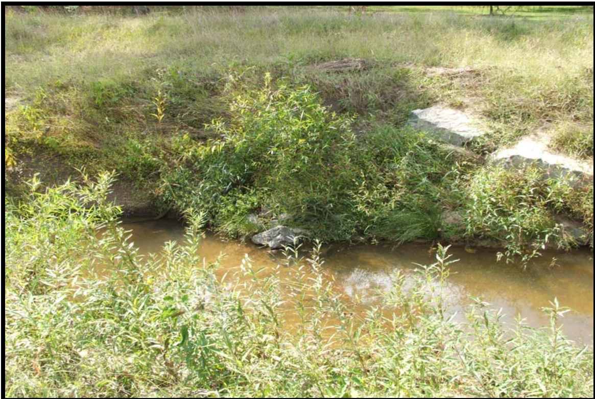
PRP 12 – Looking at 15' CMP coming into Third Fork Creek; pipe is obscured from view because of vegetation.
