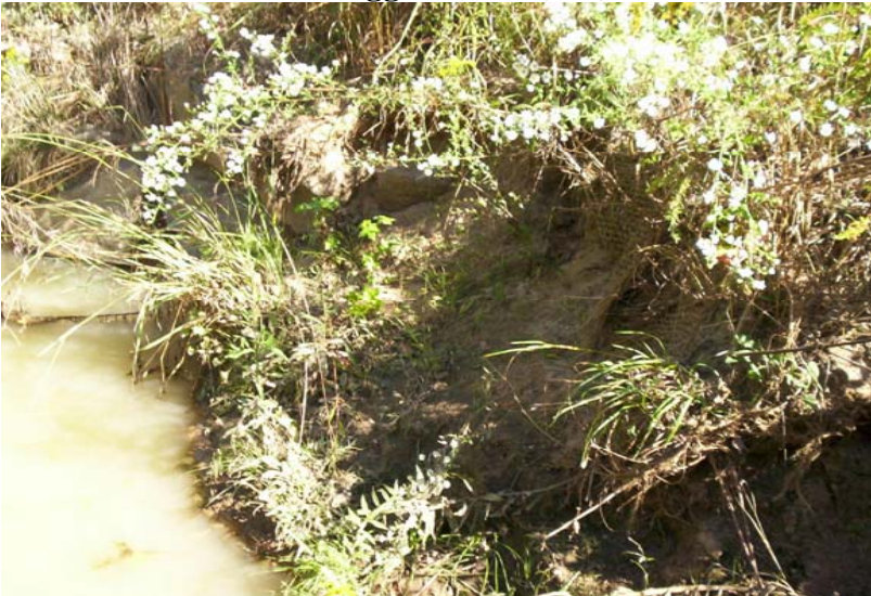
SP3. Bank Undercut/Slump
