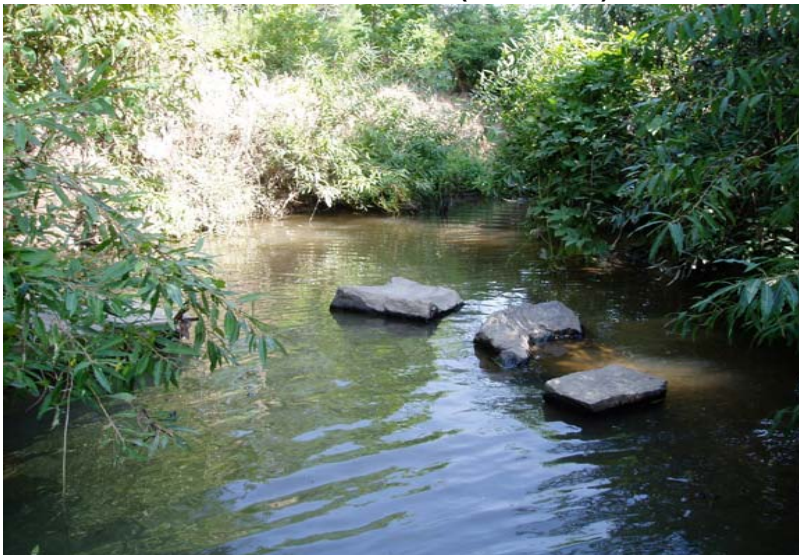
SP7-Structure not holding grade (10/28/2008)
