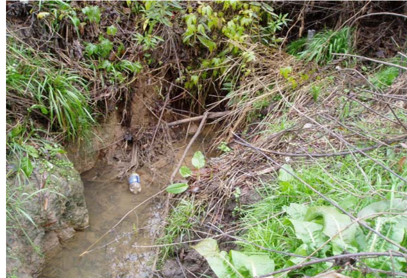
SP2-Headcut in UT/Stormwater (10/28/2008)
