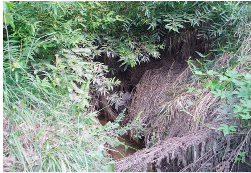
SP2-Headcut in UT/Stormwater (7/17/2009)
