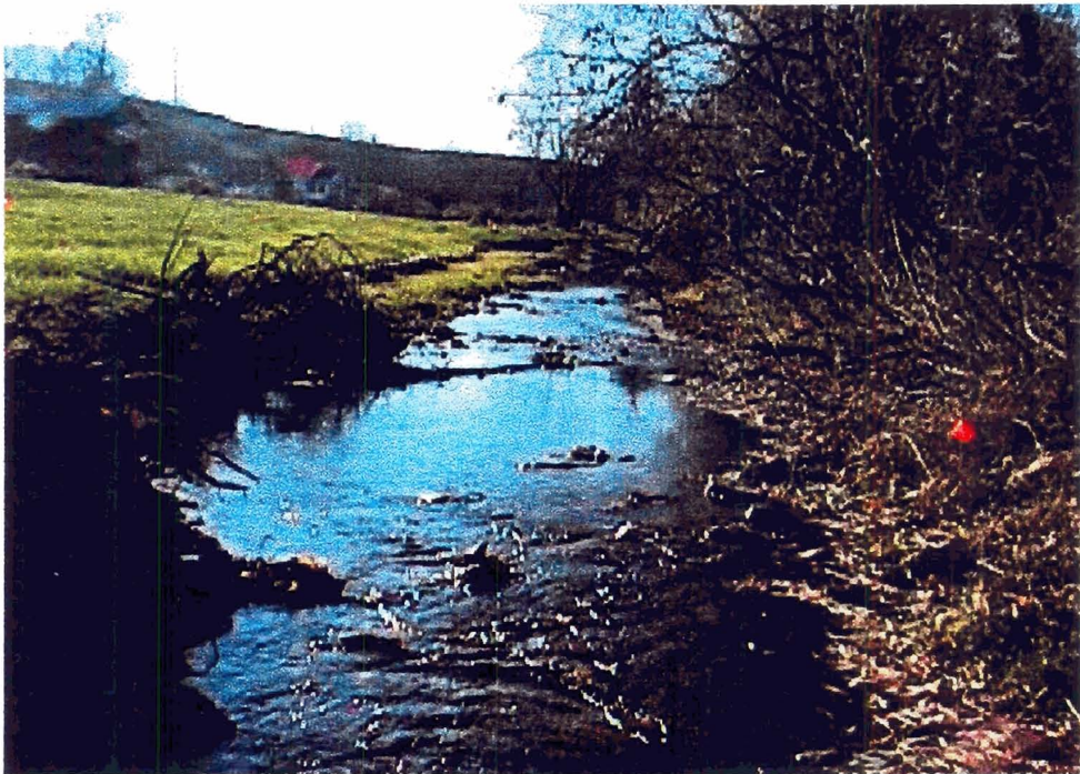
Downstream photo of same location showing lower rootwad revetment and banks before and after construction
