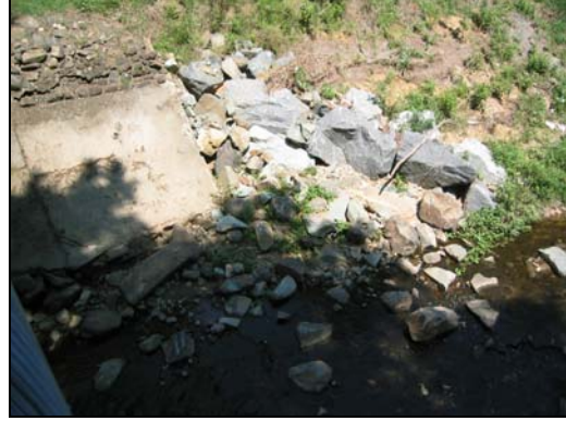
Issue Photo 2. Near Station 36+50. Potential scour at bridge abutment.
