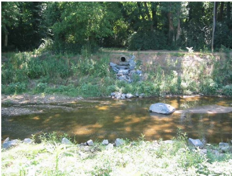
P16. Below XSC-7 Left Bank (Station 30+80)
