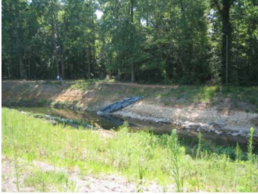
Issue Photo 1. Near Station 28+50. Poor vegetation establishment along the stream bank.
