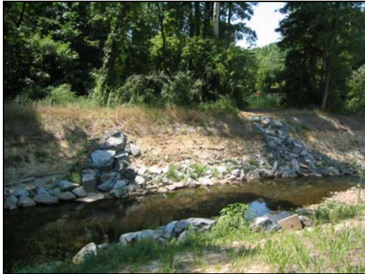
Issue Photo 3. Near Station 43+00. Poor vegetation establishment along the stream bank.
