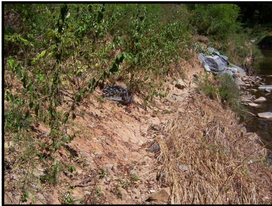
Photo 3—Typical Bank Scour
