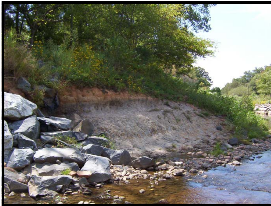
Photo 1— Typical Bank Scour
