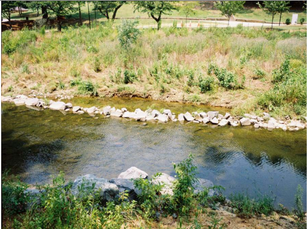
SP 2: Scour behind boulder toe protection
