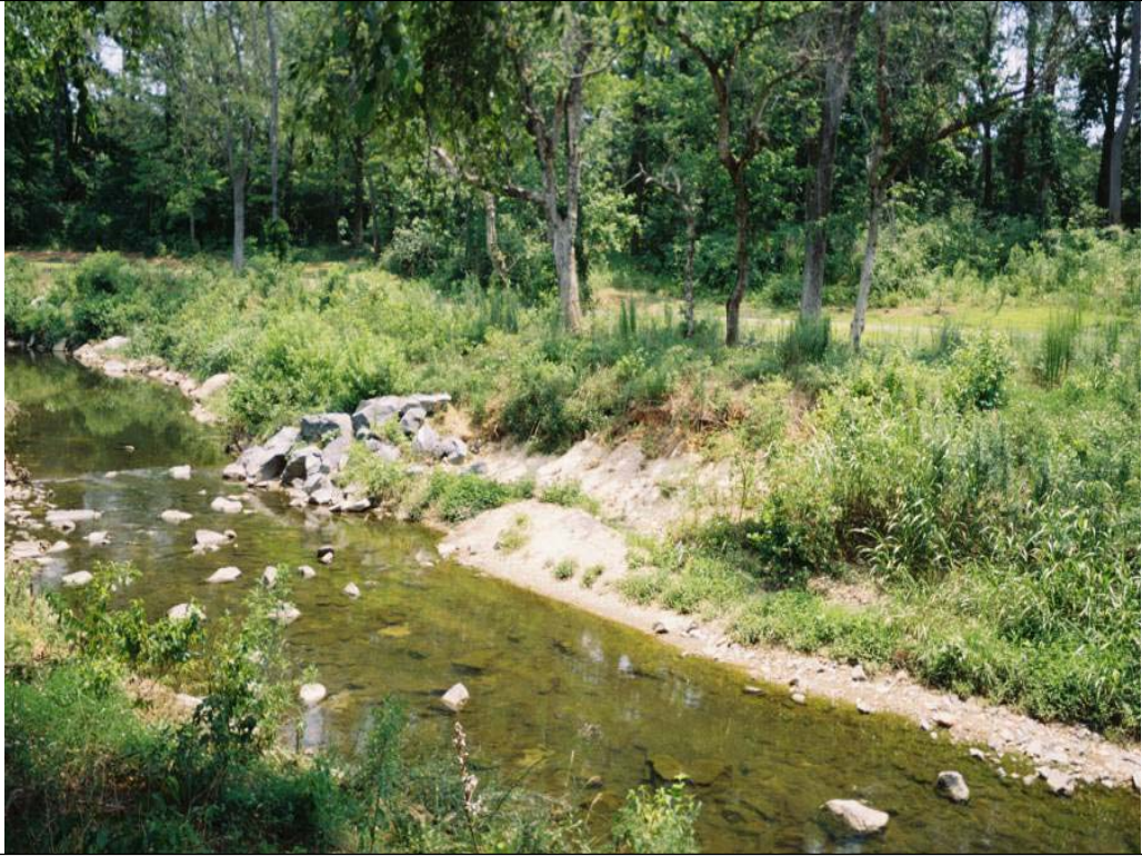
SP 5: Scour on left bank
