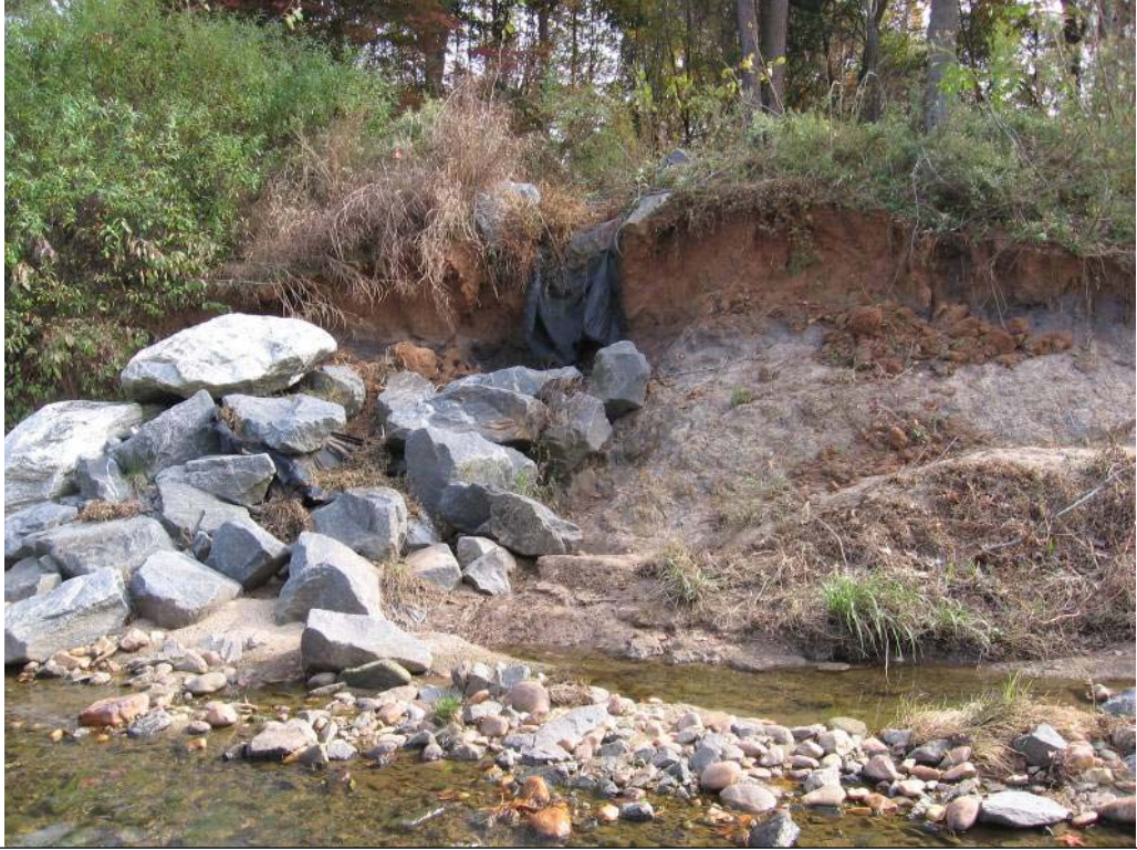
SP 1: Scout on left bank with failing rock stabilization
