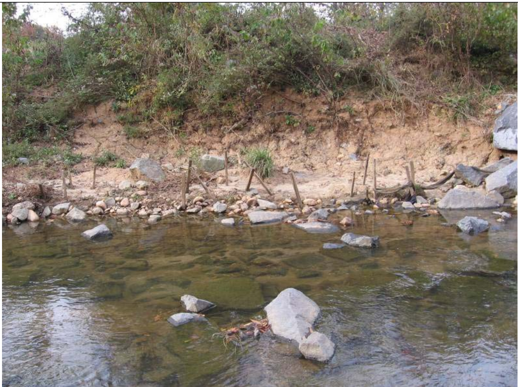
SP 6: Scour on Right Bank
