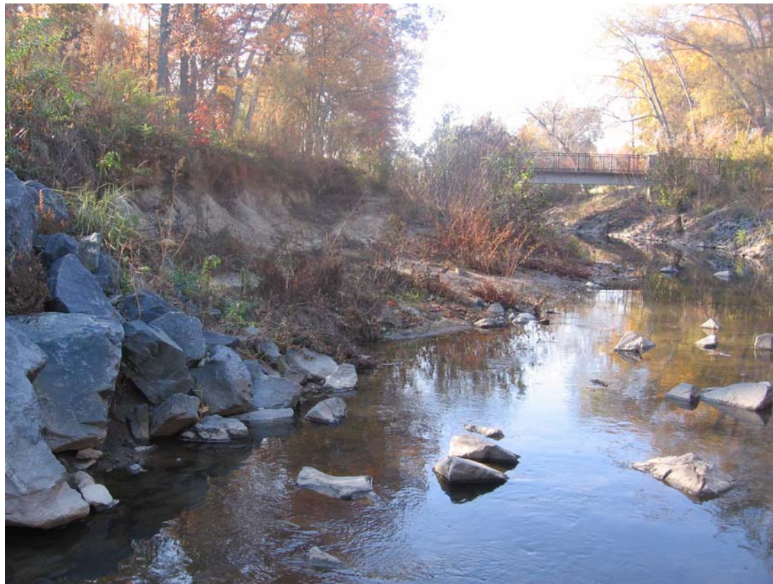
SP 3: Looking downstream at left bank, scour
