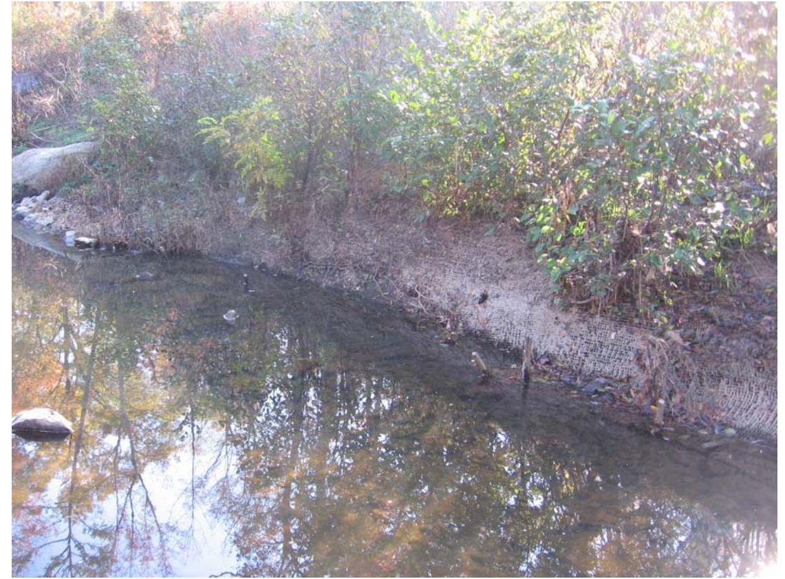
SP 2 : Looking at right bank, bank scour behind coir log
