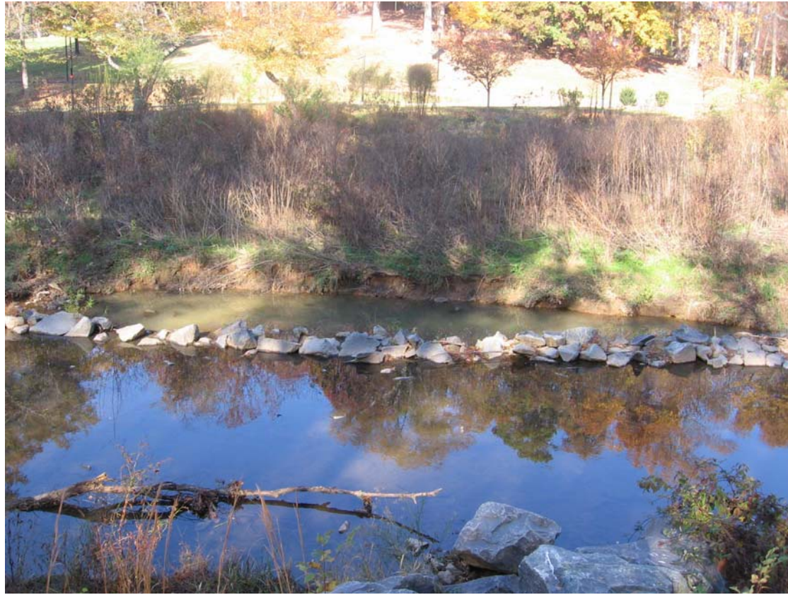
SP 5: Looking at right bank, scour behind boulder toe protection
