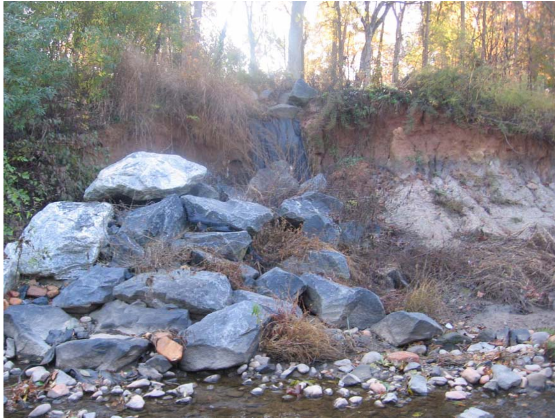
SP 1: Looking at left bank, collapsed structure
